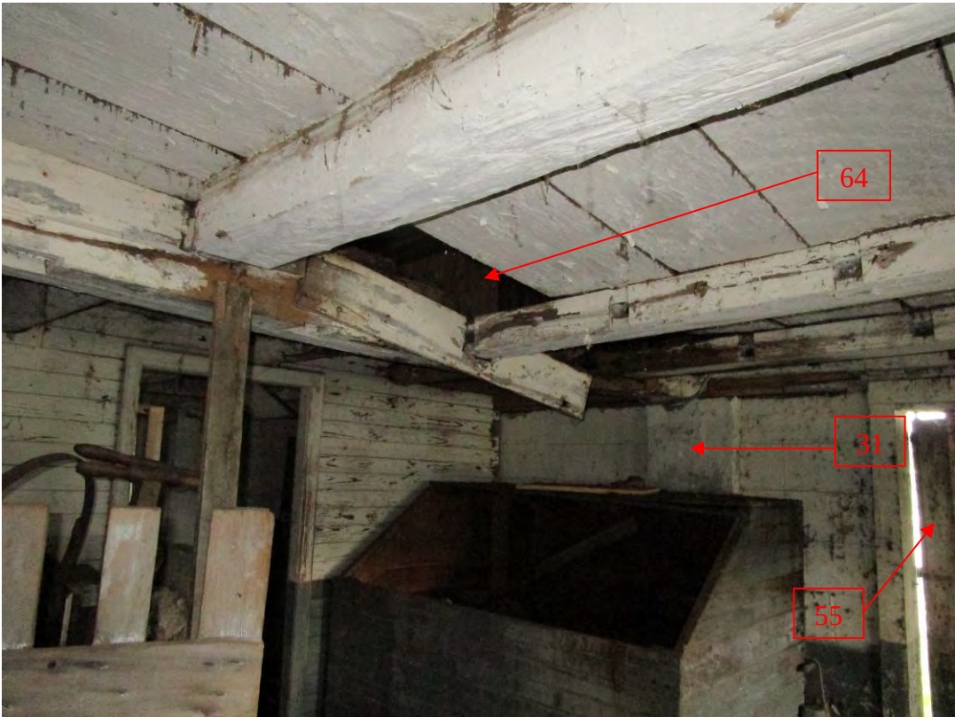
Floor Failure Northwest Corner
