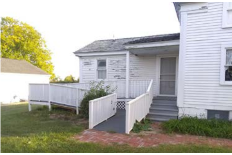
Deferred Maintenance at Cranson-Hinbern House
