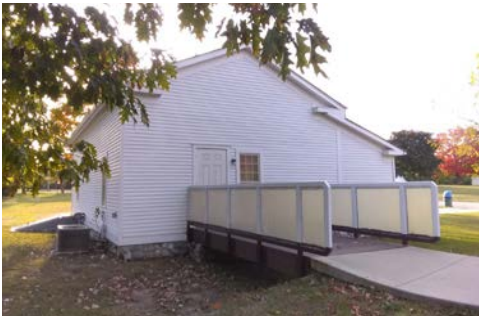
Example of ADA enhancement opportunity
