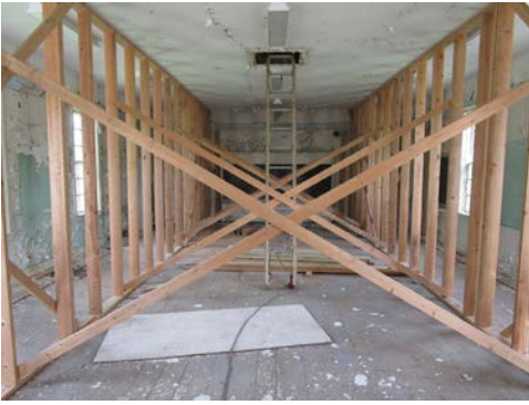
Interior Bracing Remaining from Building Move
