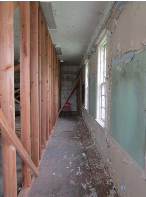
Flacking Paint on Eastern Interior Wall
