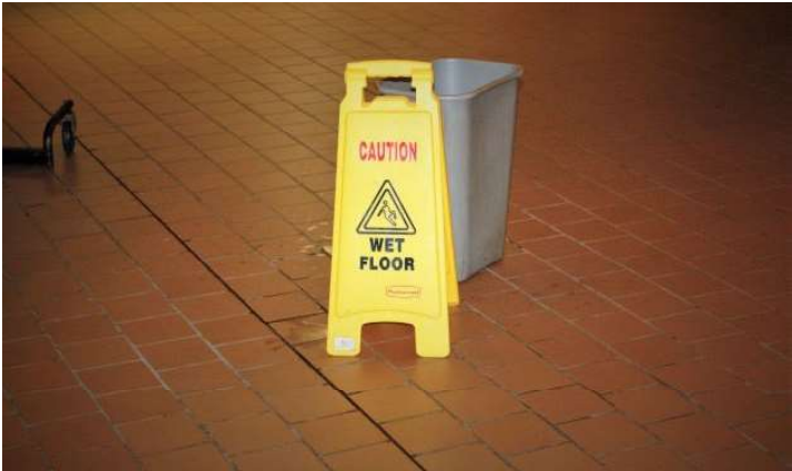
First Floor Leak
