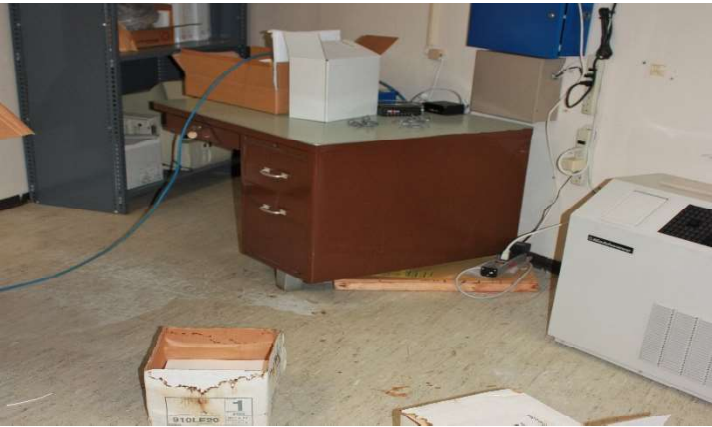
Phone Room Leak Aftermath
