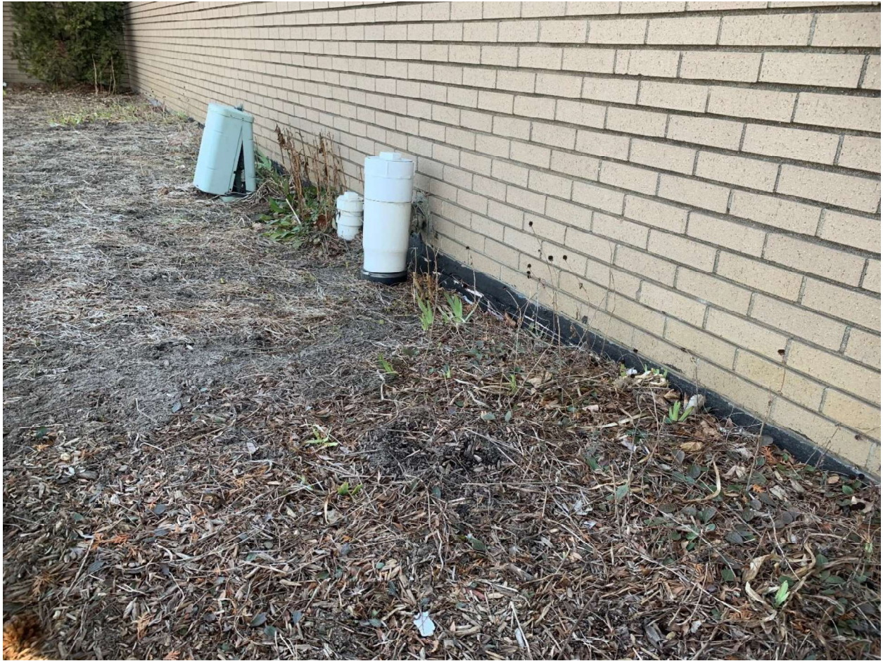
Figure 18 Grade settled along foundation
