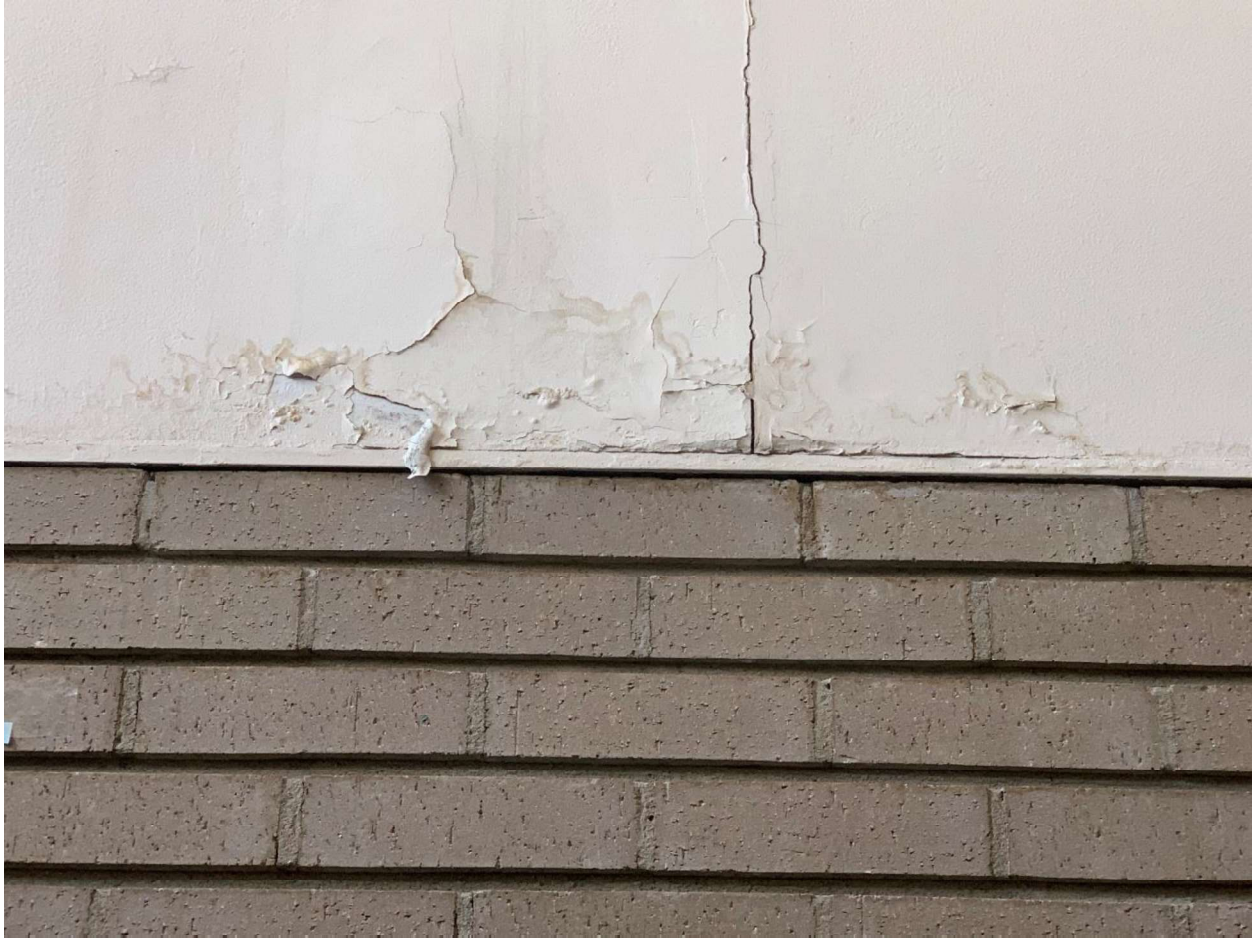
Figure 20 Water damaged drywall main floor
