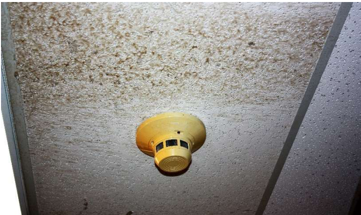
Basement Leak Near Elevator 2016
