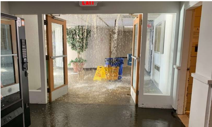
Ruptured Pipe in Annex 2022
