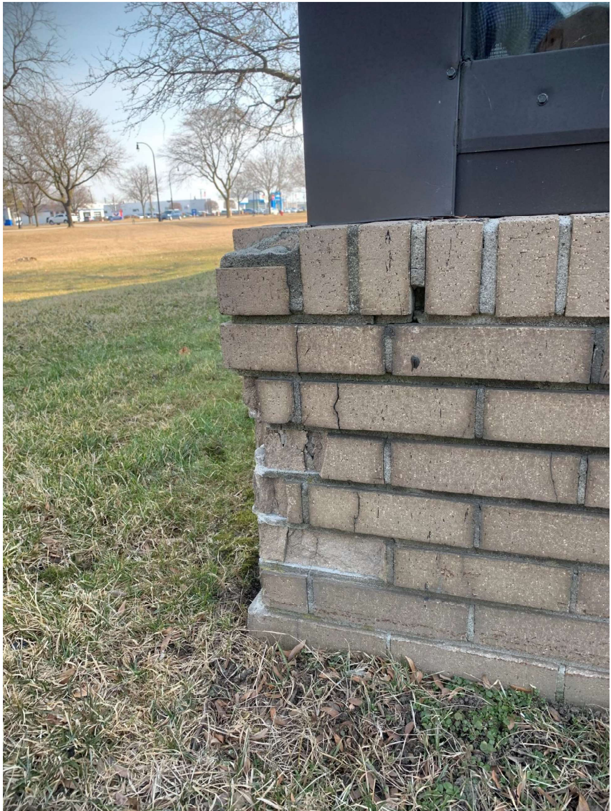
Figure 1 damaged brick and mortar from water
