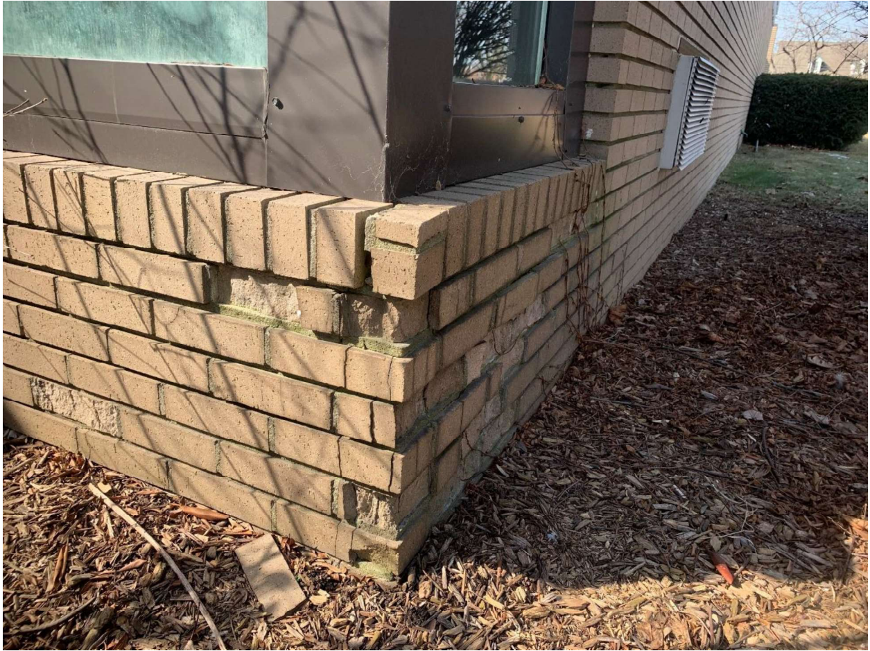
Figure 2 Brick and mortar damaged from water infiltration
