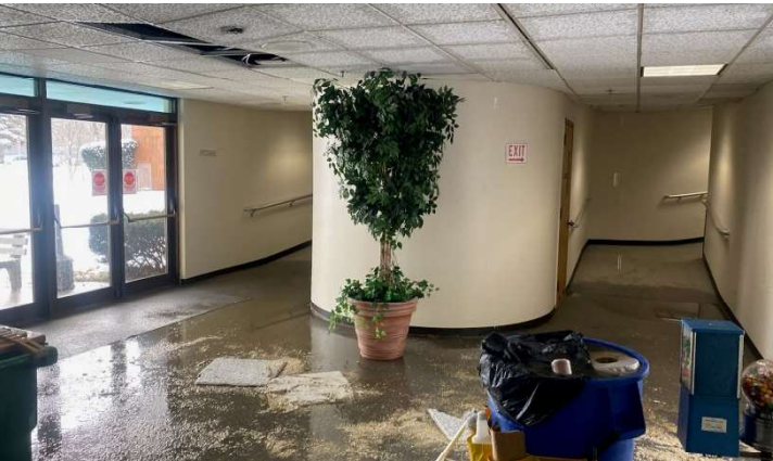
Annex Hall Damage 2022
