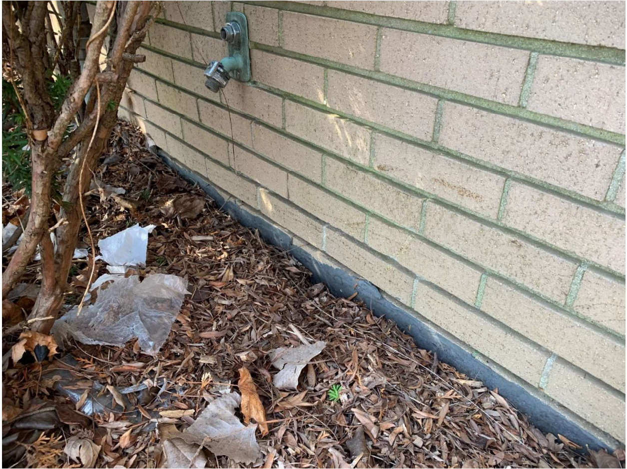
Figure 19 Grade settled along foundation
