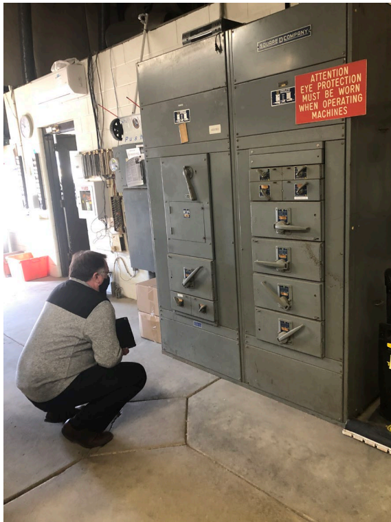
Figure 4: Existing electrical equipment and configuration
