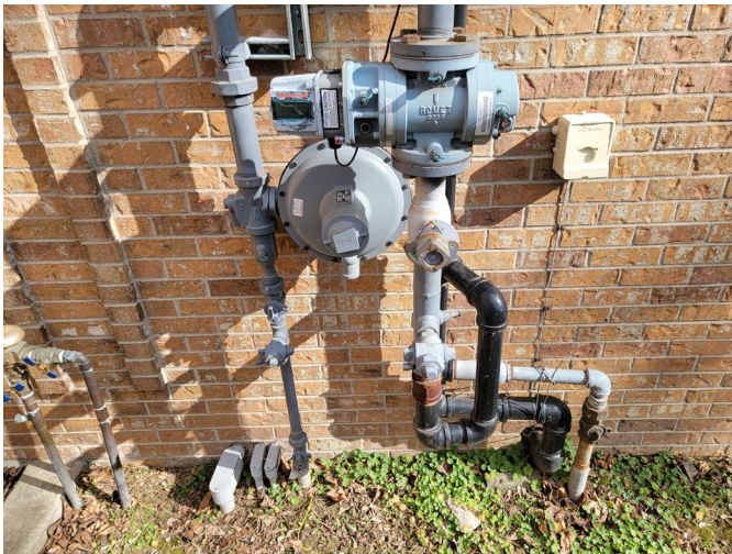
Figure 7: Existing NG Services – Side of Building
