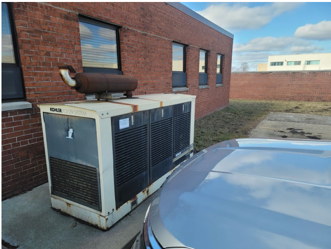
Figure 5: Existing NG Generator 50 kW
