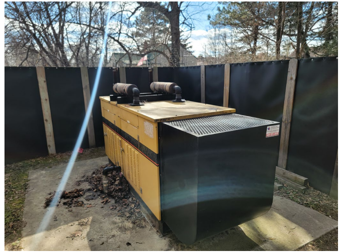
Figure 3: Existing NG Generator
