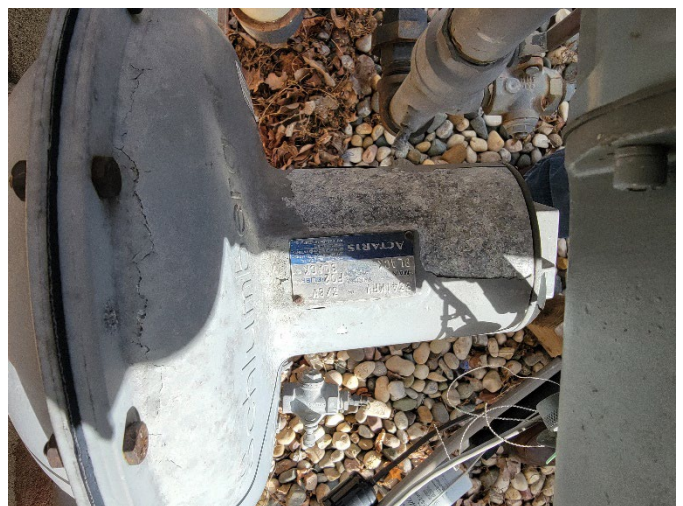
Figure 9: Existing NG Generator Regulator Tag
