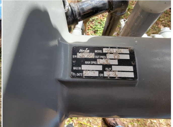
Figure 8: Existing NG Pressure Regulator
