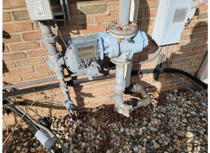
Figure 7: Existing NG Meter / Regulator Assembly
