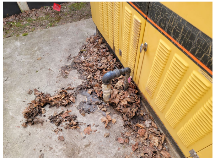
Figure 5: Existing NG Up from Below Grade to Existing NG Generator
