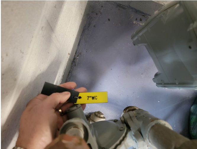
Figure 11: Existing NG Regulator Pressure Tag
