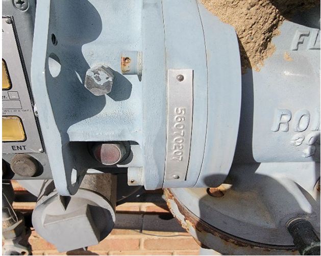
Figure 10: Existing NG Generator Meter Tag
