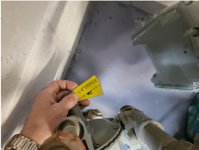
Figure 12: Existing NG Regulator Orifice Tag
