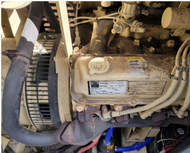
Figure 6: Existing NG Generator 100 kW Motor
