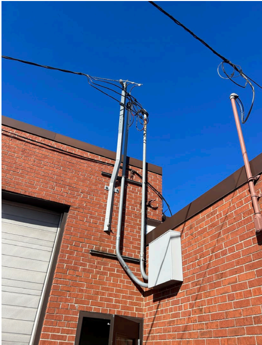
Figure 2: Overhead service to building
