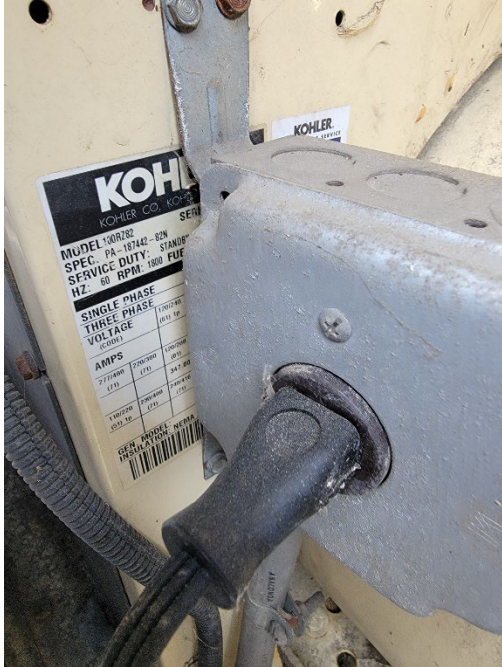
Figure 5: Existing NG Generator 100kW Tag
