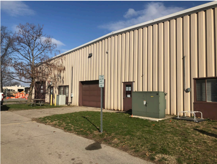
Figure 3: Existing transformer along south façade (possible location)
