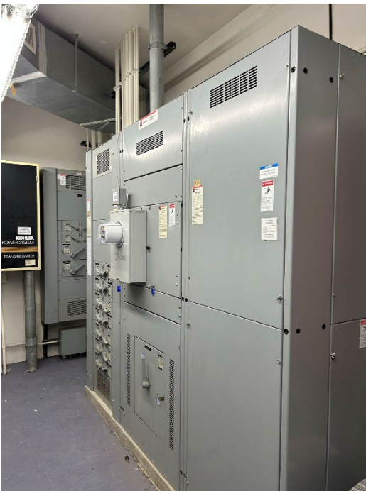
Figure 2: Existing MDP, transfer switch and EDP
