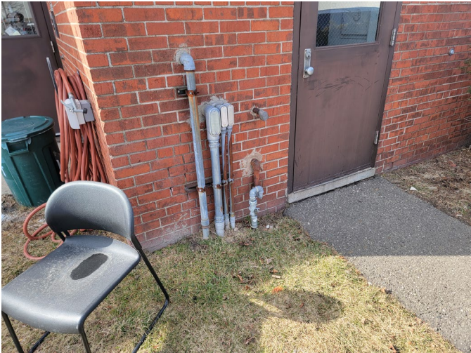
Figure 9: Existing NG Piping that Goes Underground to Exiting NG Generator
