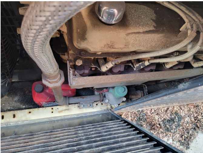
Figure 8: Existing NG Incoming Piping (From Underground)
