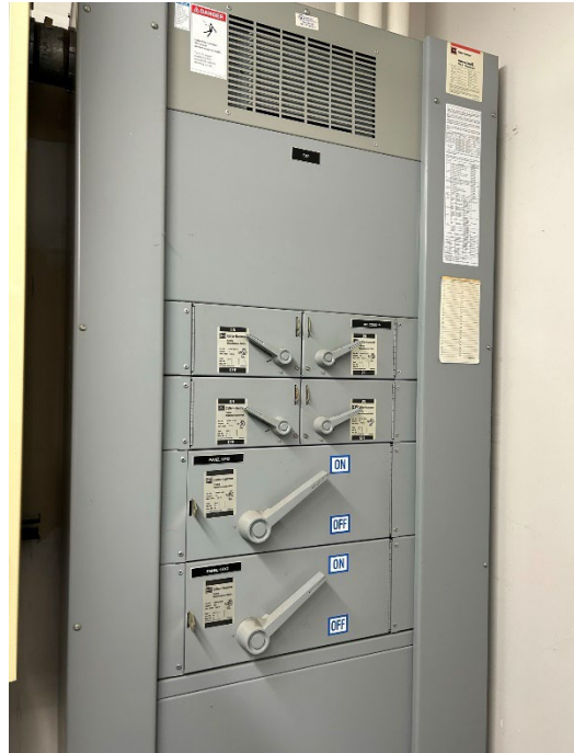
Figure 3: Existing Emergency Distribution Panel
