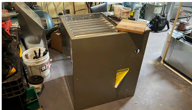
New HVAC equipment
