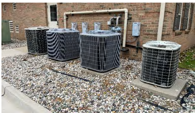
Air conditioning units
