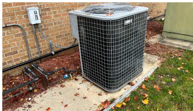
Air conditioning unit
