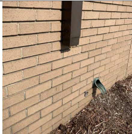
Reinstall proper termination of downspouts, regrade low spots that have settled due to water.
