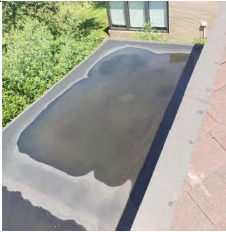
Roof ponding, little/no positive slope to scuppers
