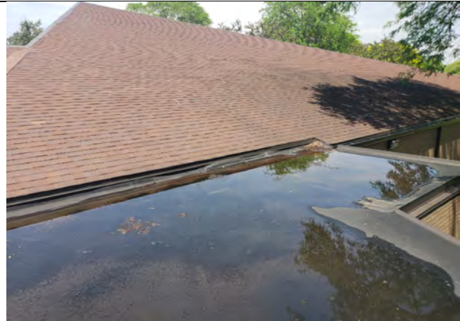
Roof ponding, little/no positive slop to scuppers. Less than minimal flashing height at transition to roof, failed flashing sealant.
