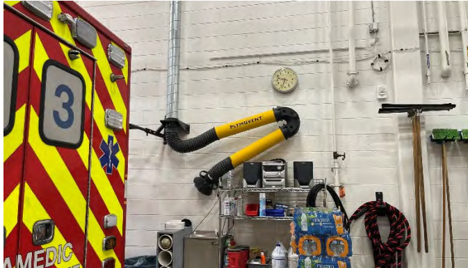
Vehicle exhaust vent
