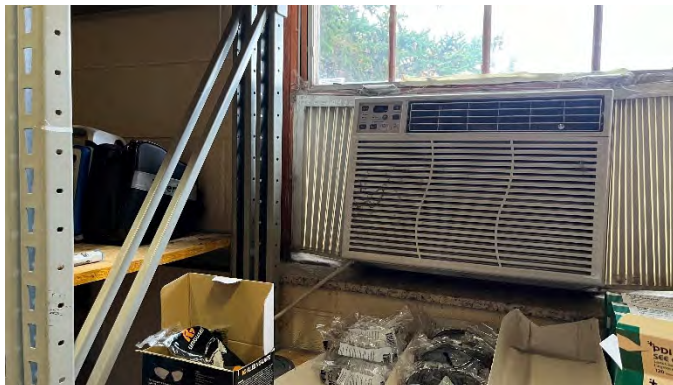
Air conditioning unit
