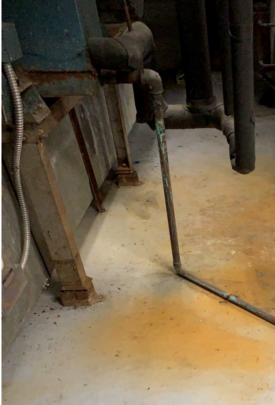
Figure 21 Furnace in basement rusting from high moisture content
