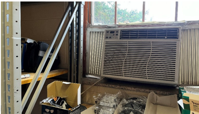
Air conditioning unit
