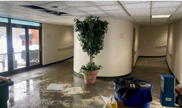
Annex Hall Damage 2022
