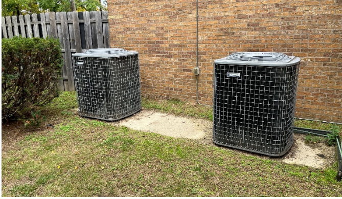
Air conditioning units
