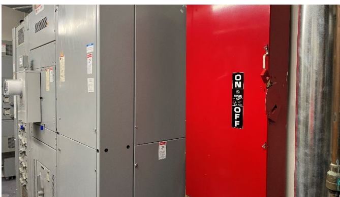
Switch gear and emergency main
