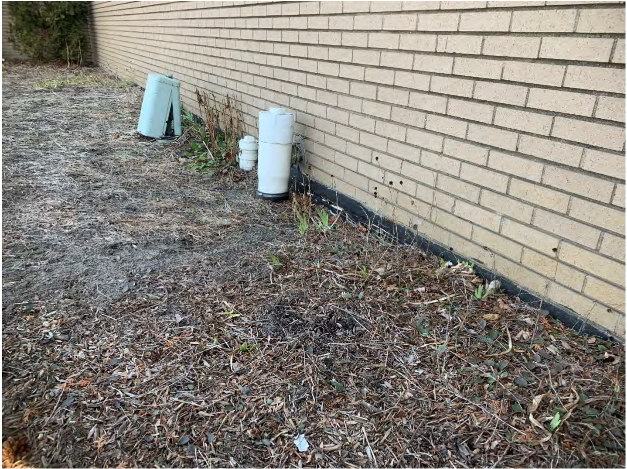
Figure 18 Grade settled along foundation
