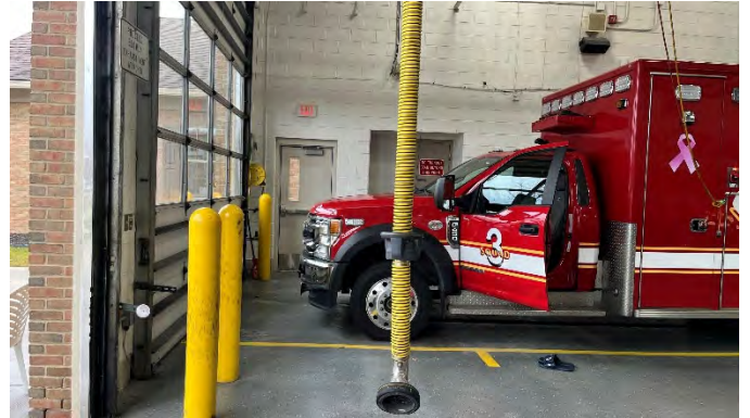
Vehicle exhaust vent
