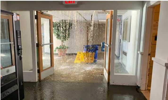
Ruptured Pipe in Annex 2022
