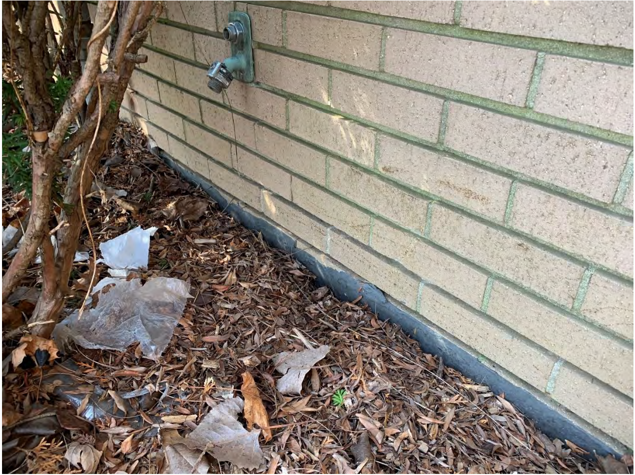
Figure 19 Grade settled along foundation
