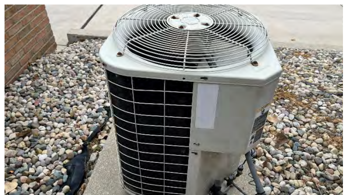
Air conditioning unit
