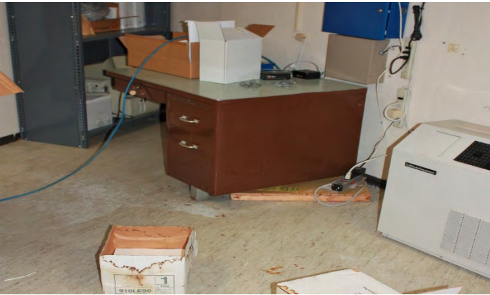
Phone Room Leak Aftermath
