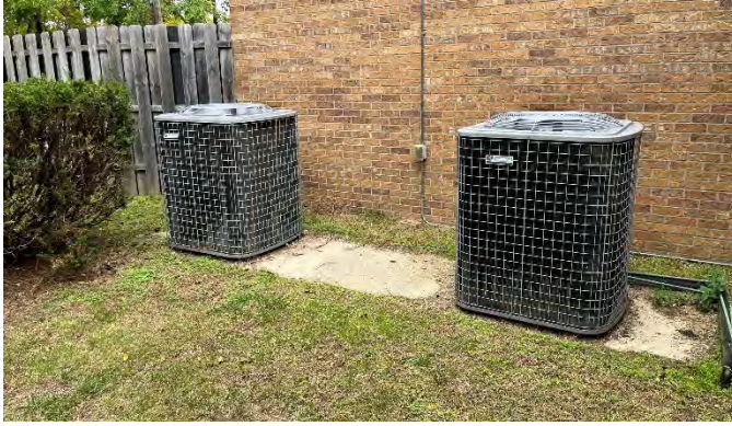
Air conditioning units
