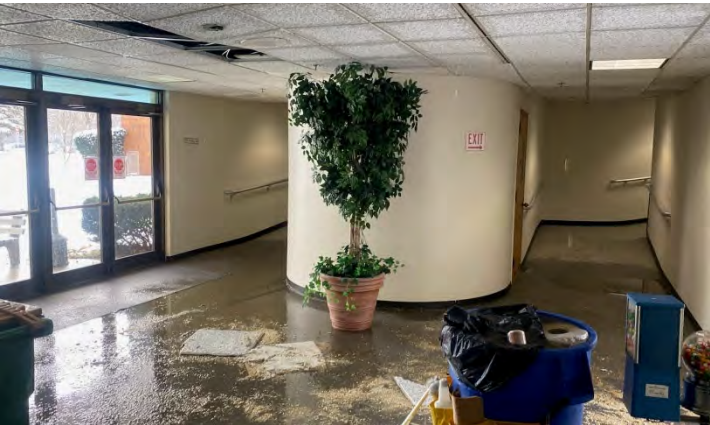
Annex Hall Damage 2022
