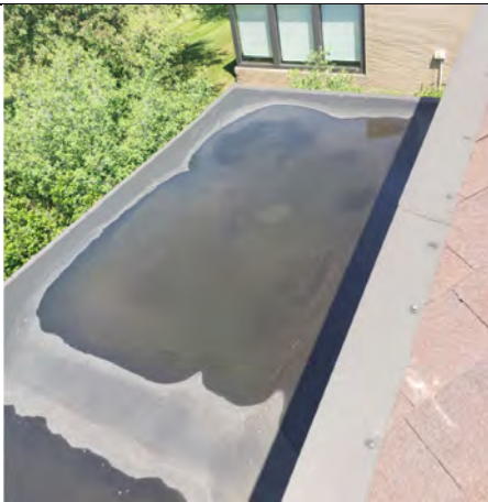
Roof ponding, little/no positive slope to scuppers
