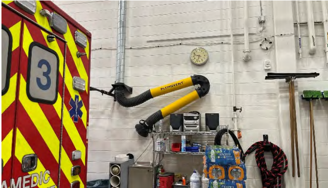
Vehicle exhaust vent
