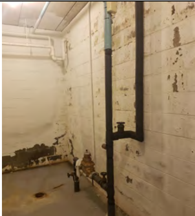
Basement, interior wall paint flaking and water infiltration from exterior.
