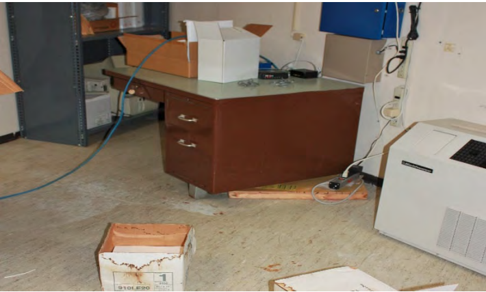
Phone Room Leak Aftermath
