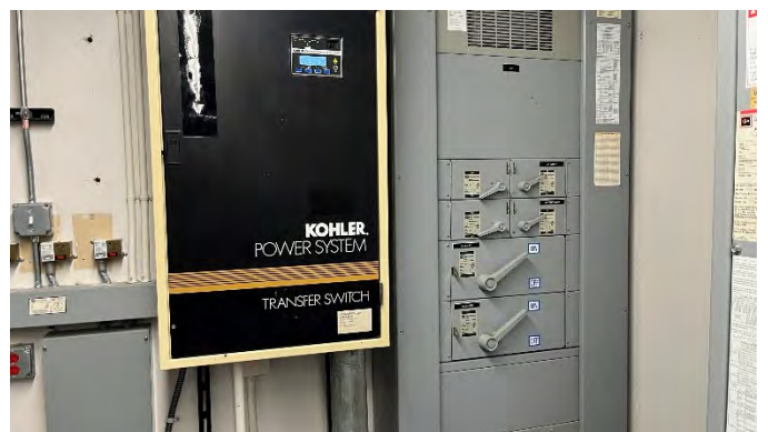
Switch gear and transfer switch
