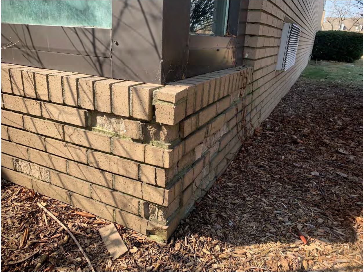
Figure 2 Brick and mortar damaged from water infiltration
