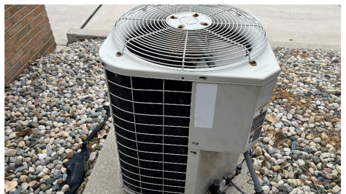
Air conditioning unit
