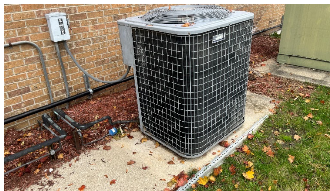
Air conditioning unit
