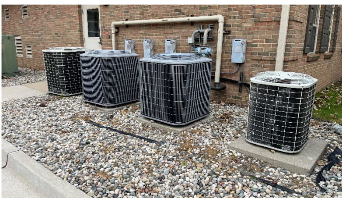
Air conditioning units
