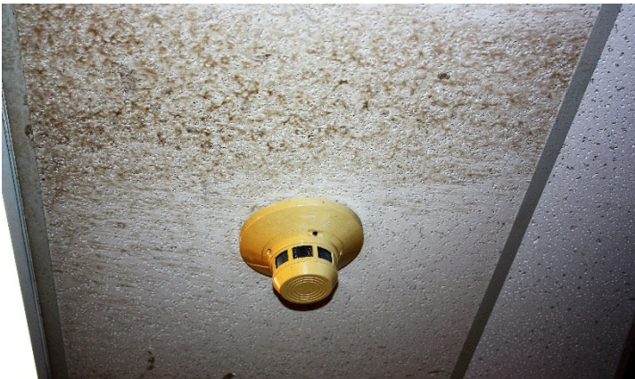
Basement Leak Near Elevator 2016
