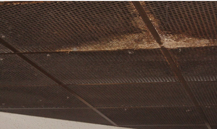
Fifth Floor Ventilation Grates 2013
