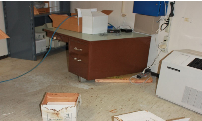
Phone Room Leak Aftermath
