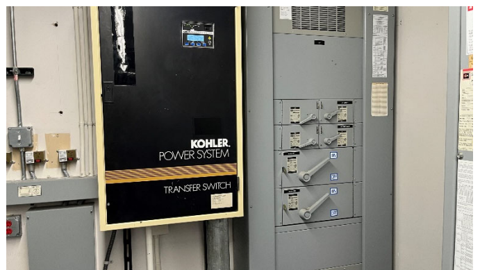
Switch gear and transfer switch
