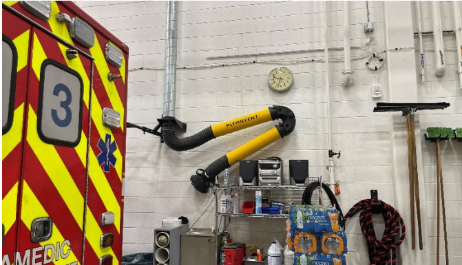
Vehicle exhaust vent
