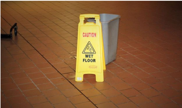
First Floor Leak
