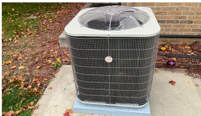
Air conditioning unit
