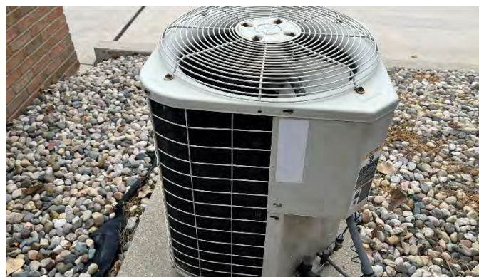
Air conditioning unit
