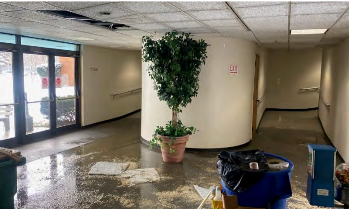
Annex Hall Damage 2022
