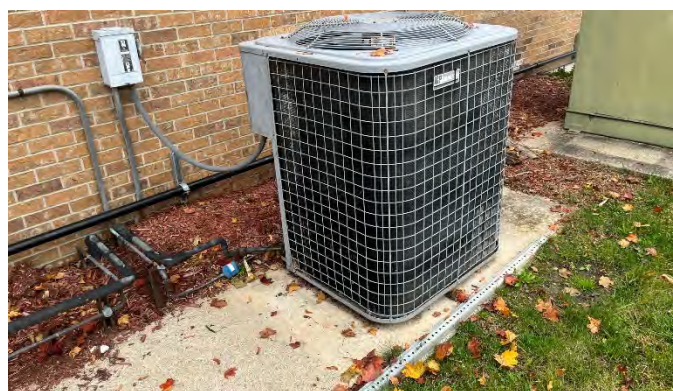
Air conditioning unit
