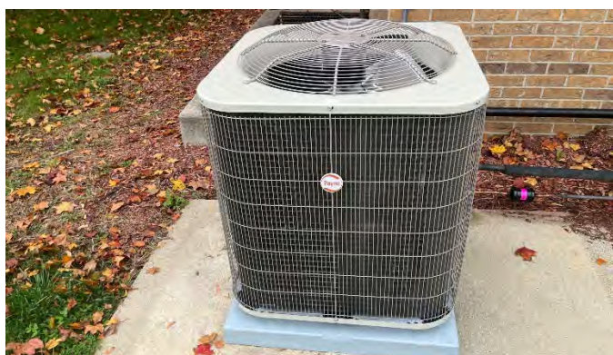
Air conditioning unit
