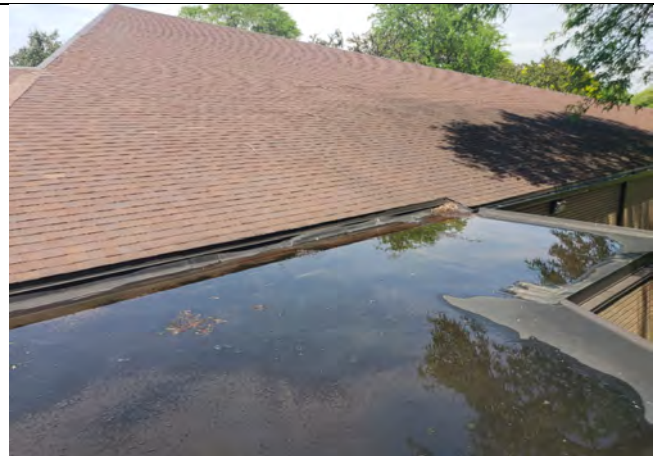
Roof ponding, little/no positive slope to scuppers. Less than minimal flashing height at transition to roof, failed flashing sealant.
