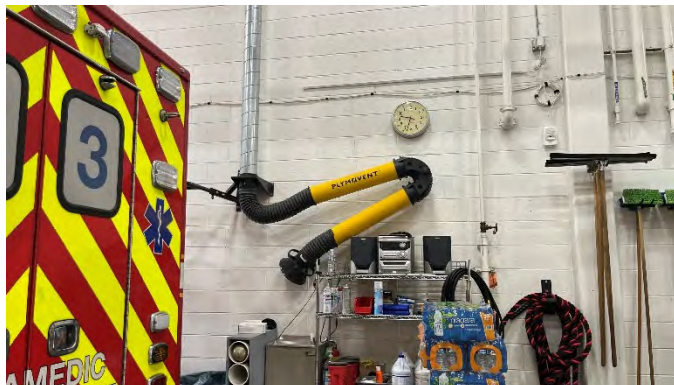
Vehicle exhaust vent
