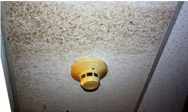
Basement Leak Near Elevator 2016
