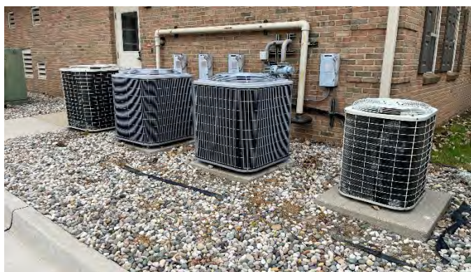
Air conditioning units
