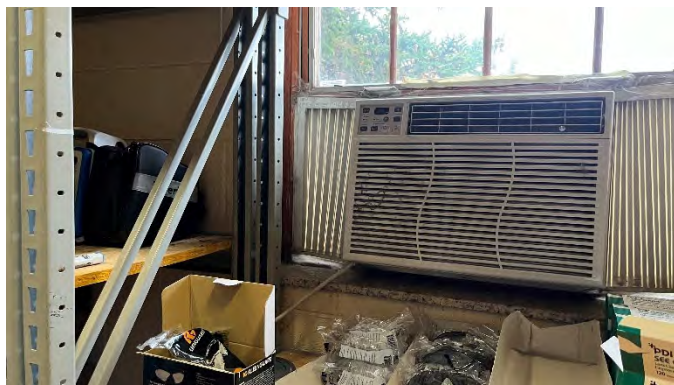
Air conditioning unit
