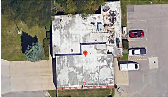
Thermoplastic Polyolefin roofing
