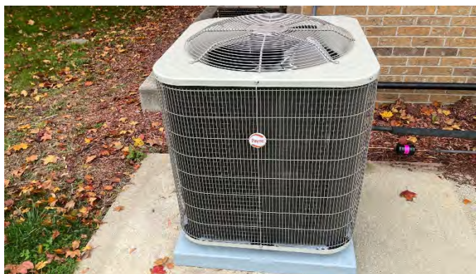
Air conditioning unit
