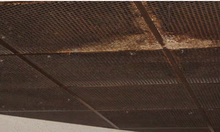
Fifth Floor Ventilation Grates 2013
