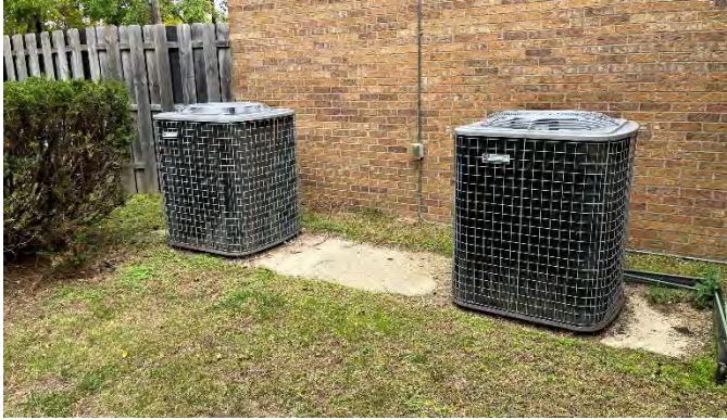
Air conditioning units
