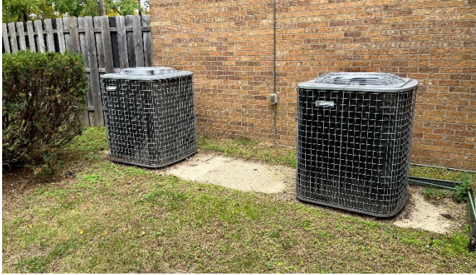
Air conditioning units
