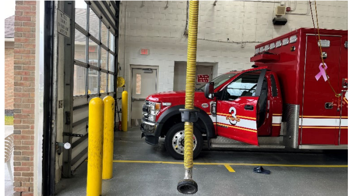
Vehicle exhaust vent
