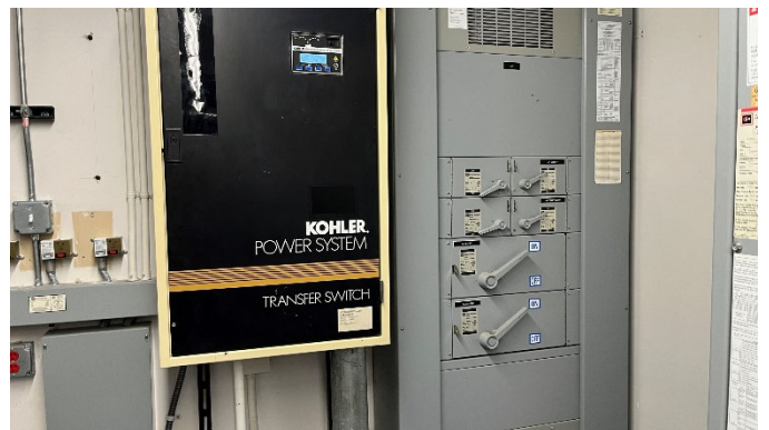
Switch gear and transfer switch
