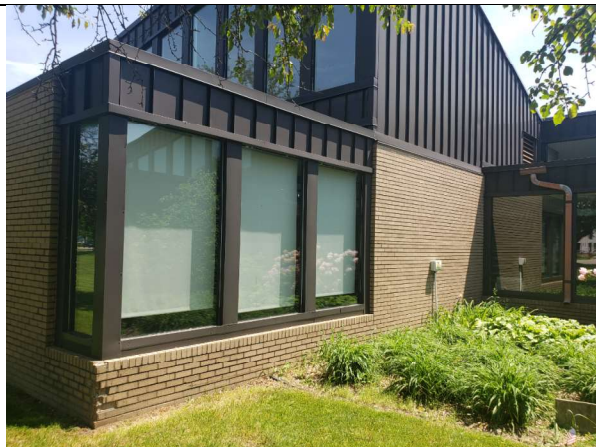
Miscellaneous brick repairs (tuckpointing), miscellaneous general window sealant failures as well as interior wood moisture issues noted in report
