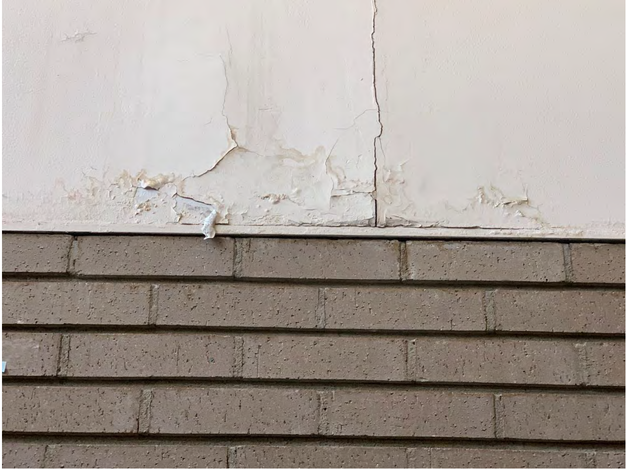
Figure 20 Water damaged drywall main floor
