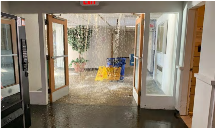
Ruptured Pipe in Annex 2022
