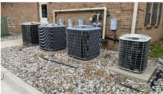
Air conditioning units
