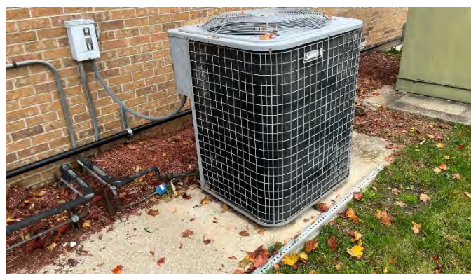
Air conditioning unit
