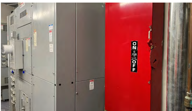
Switch gear and emergency main
