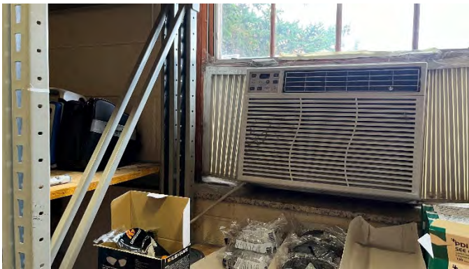
Air conditioning unit
