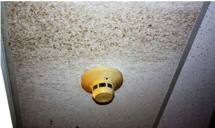
Basement Leak Near Elevator 2016
