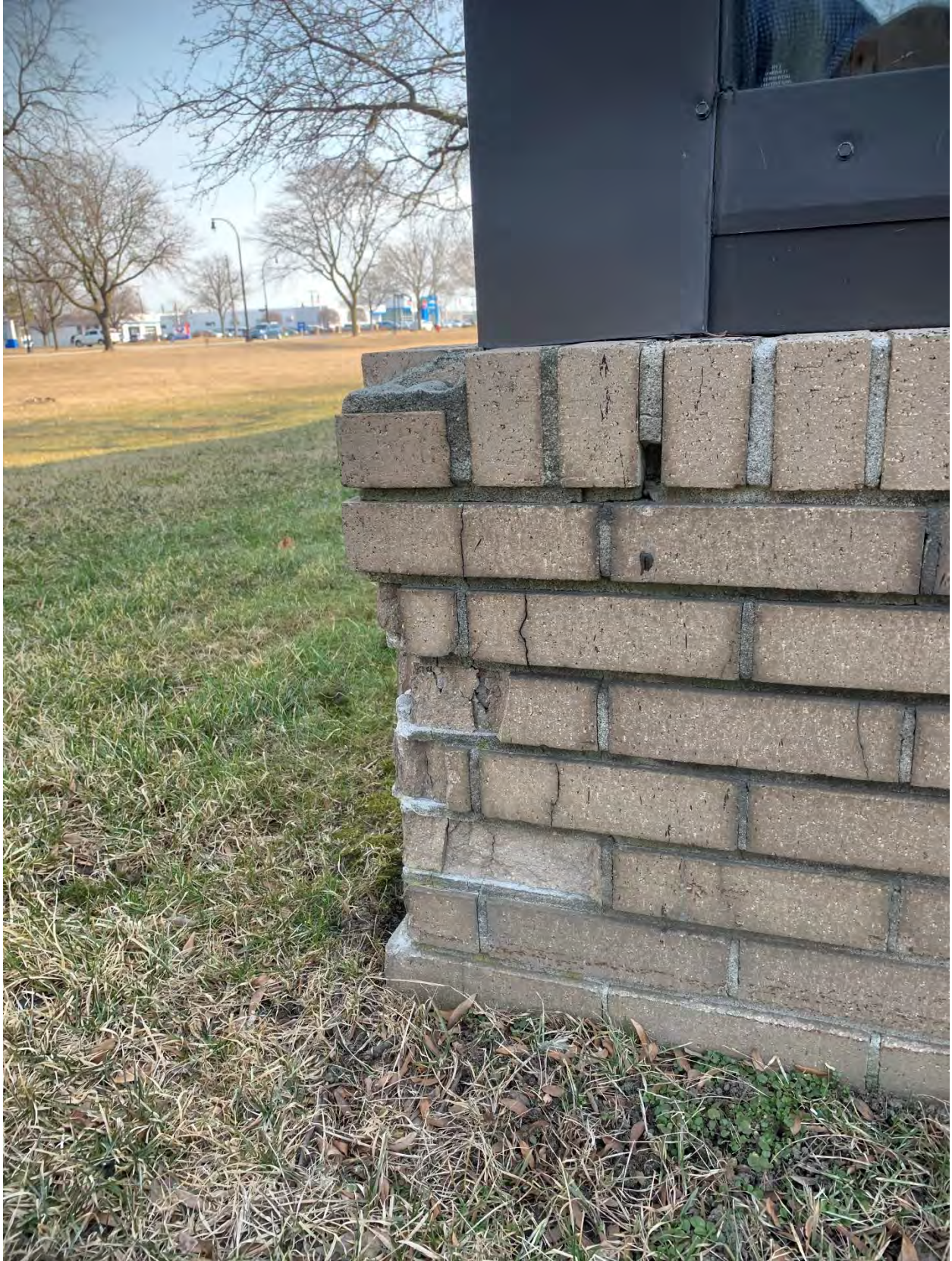
Figure 1 damaged brick and mortar from water
