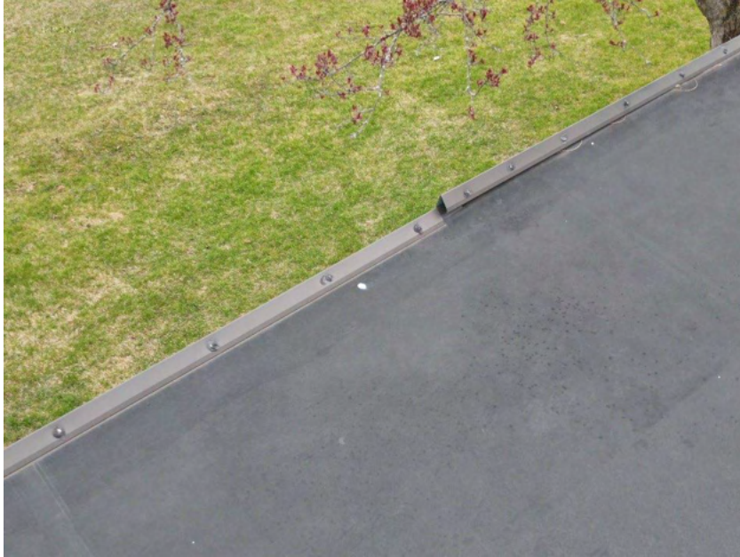
Flat Roof – Loose flash panel (Plymouth Rd Photo No. 33)
