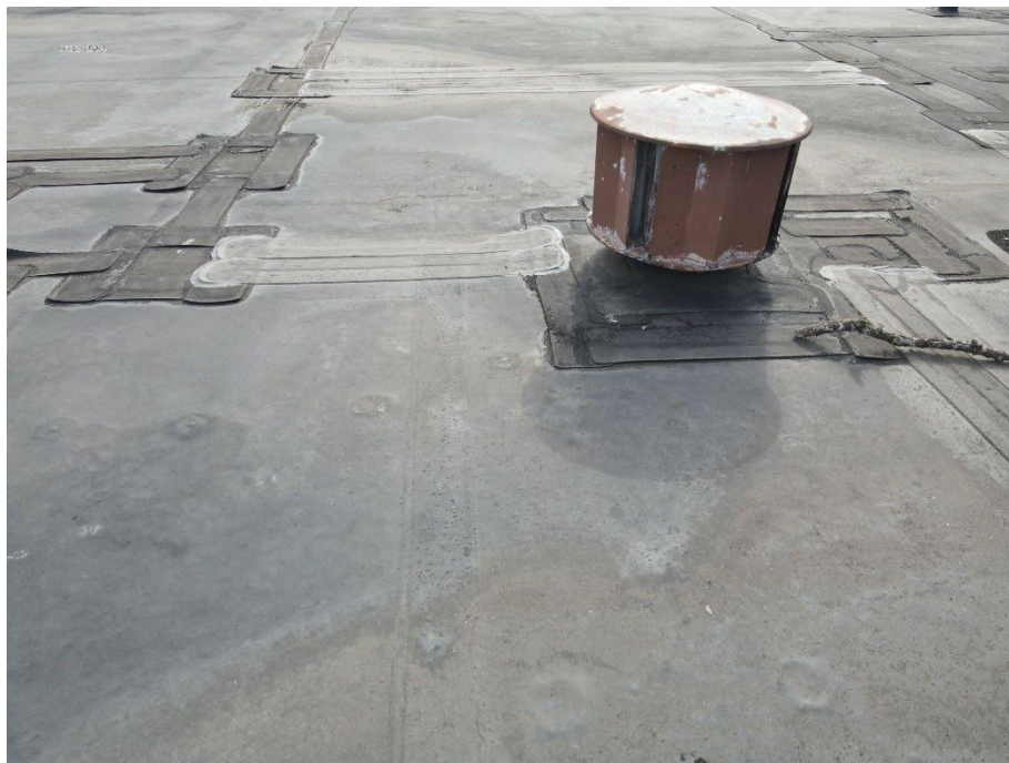
Flat Roof – Damage of patching (Woodring Ave Photo No. 8)
