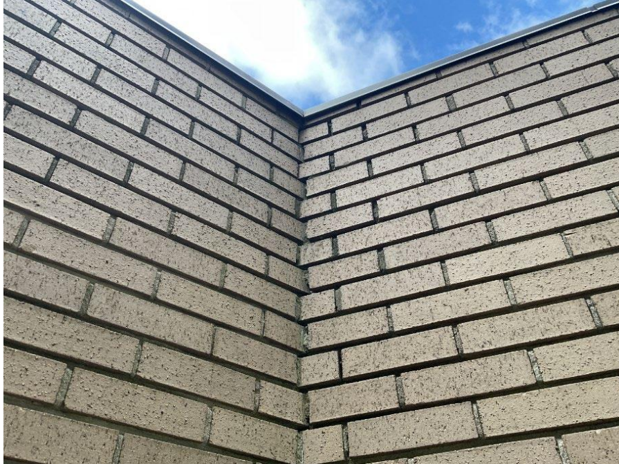
Exterior Wall – Mortar damage (Photo No. 5008)
