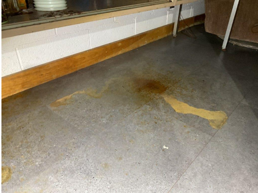
Main Floor Lounge Room – Water mark on floor (Photo No. 4831)
