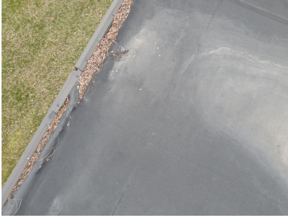
Flat Roof – Holes at edge (Plymouth Rd Photo No. 15)
