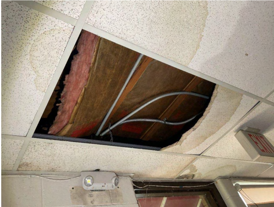
Main Floor Work Room Ceiling - Water damage (Photo No. 4804)
