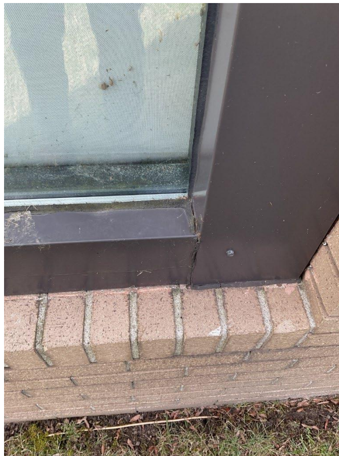
Exterior - Window seal damage (Photo No. 5022)
