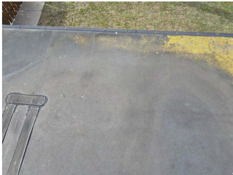
Flat Roof – Damage at patching (Parking Lot Side Photo No. 39)
