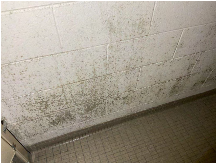
Basement Wall – Mold (Photo No. 4719)
