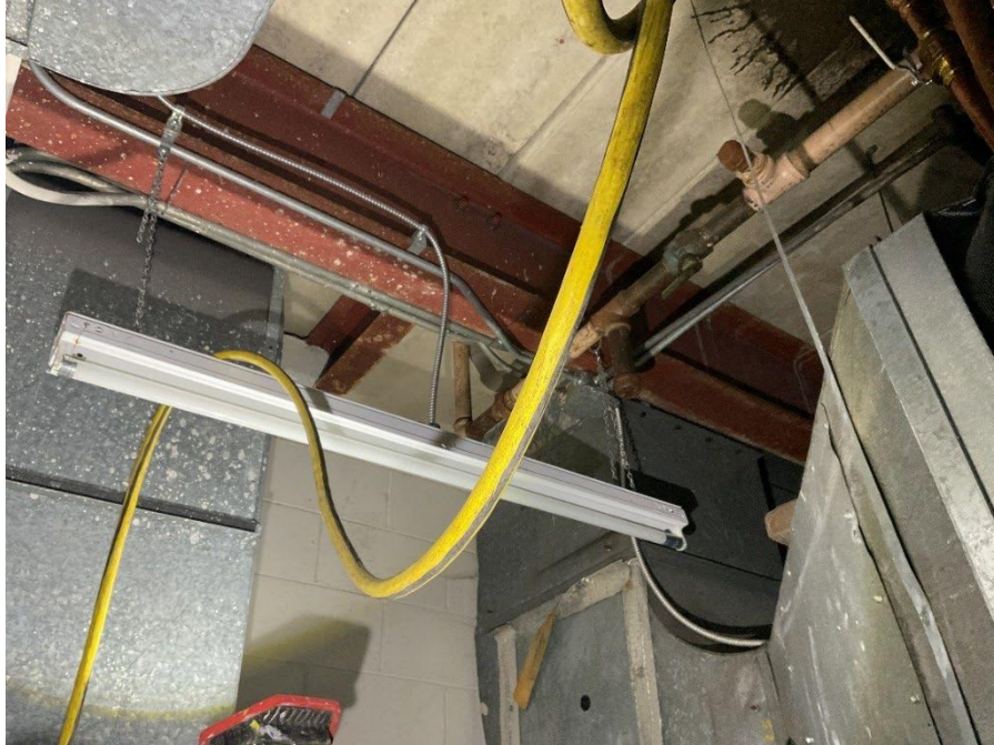
Basement – Steel beam corrosion (Photo No. 4733)
