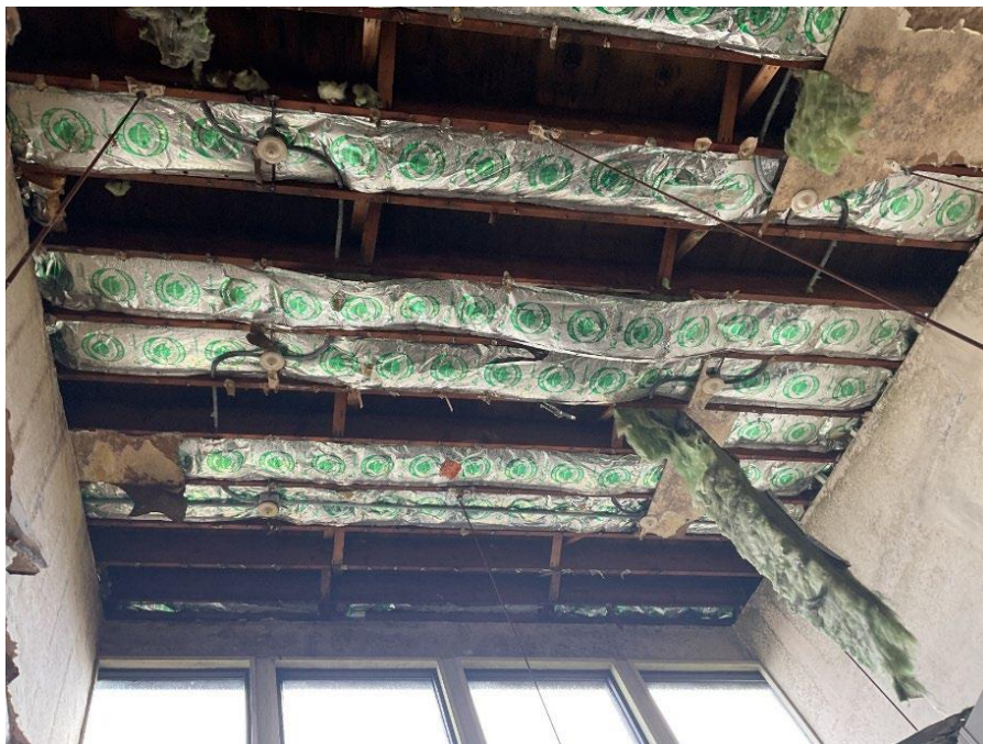
Main Floor - Ceiling damage/ insulation damage/ mold (Photo No. 4903)
