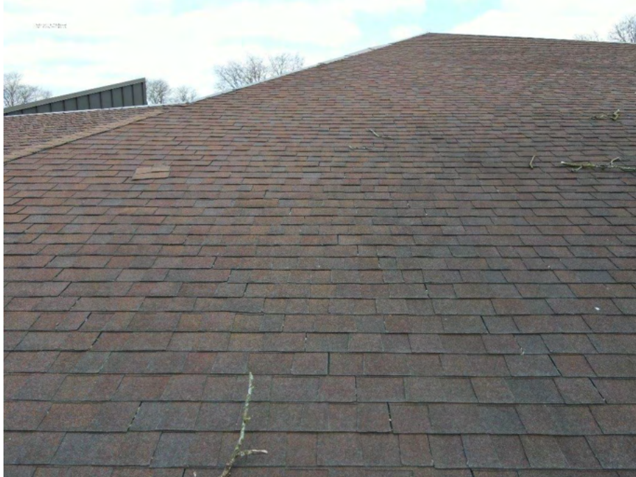
Shingle Roof – Loose piece (Loveland St and Parking Lot Photo No. 1)
