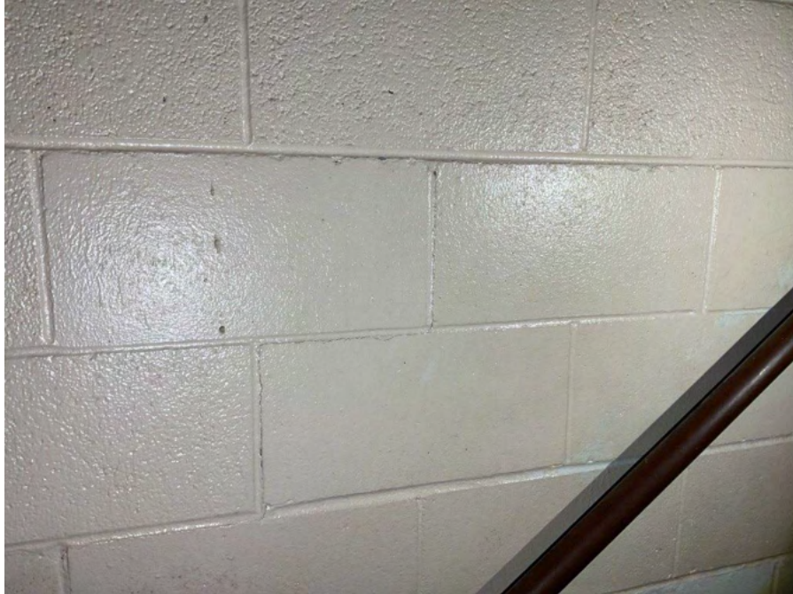
Stair Well – wall cracks/rusty handrail (Photo No. 4749)
