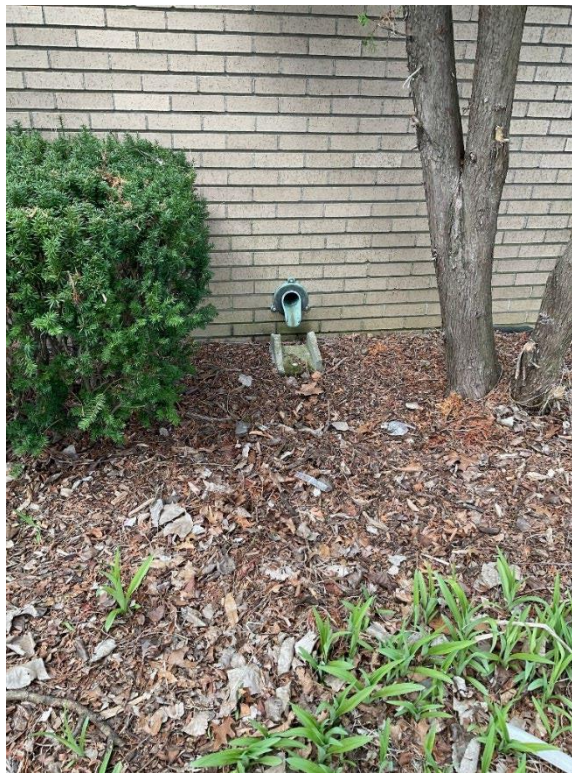
External Area - Down spout drain with no positive drain on ground (Photo No. 5007)
