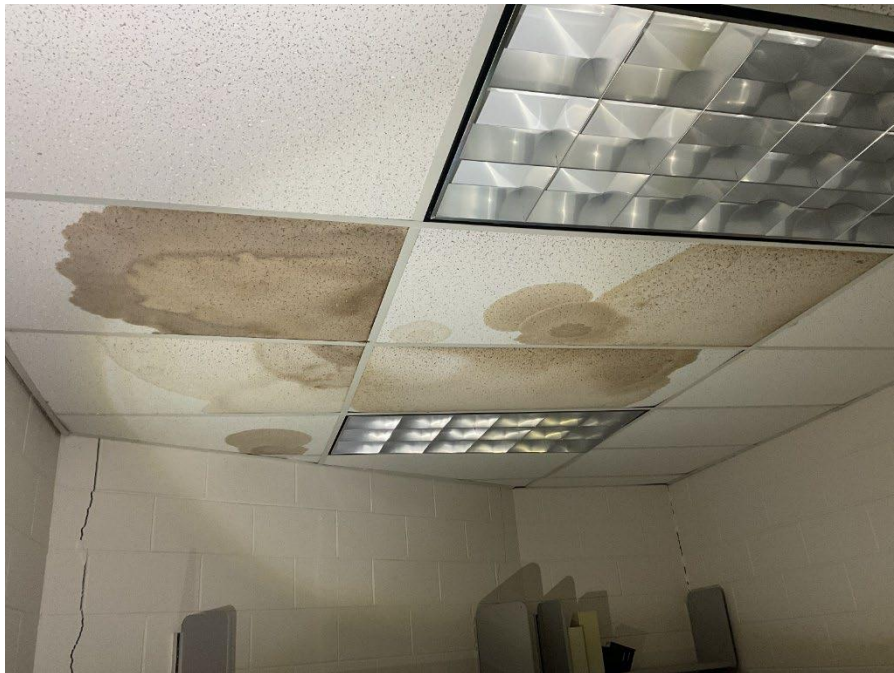
Main Floor – Librarian Room – Cracks on wall/ water damage on ceiling (Photo No. 4822)
