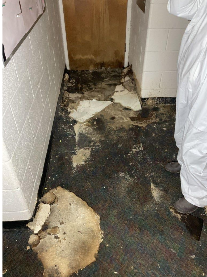
Main Floor Carpet – Mold and stockpiled with ceiling material (Photo No. 4784)
