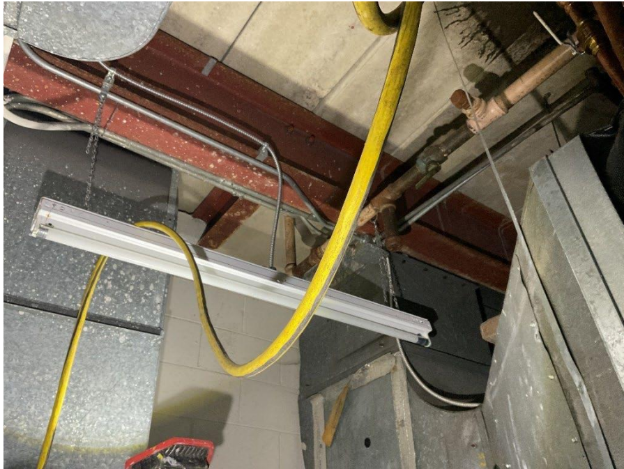
Basement – Steel beam corrosion (Photo No. 4733)
