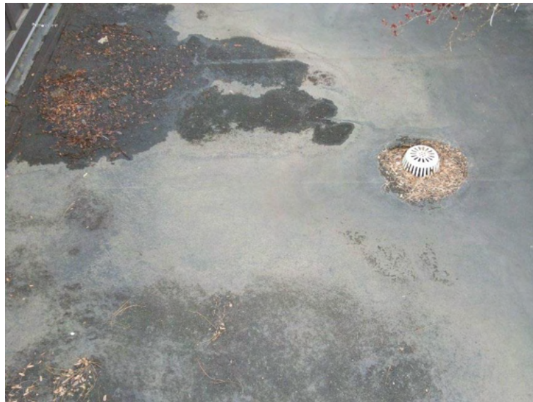
Flat Roof – Lack of positive drain (Parking Lot Side Photo No. 20)
