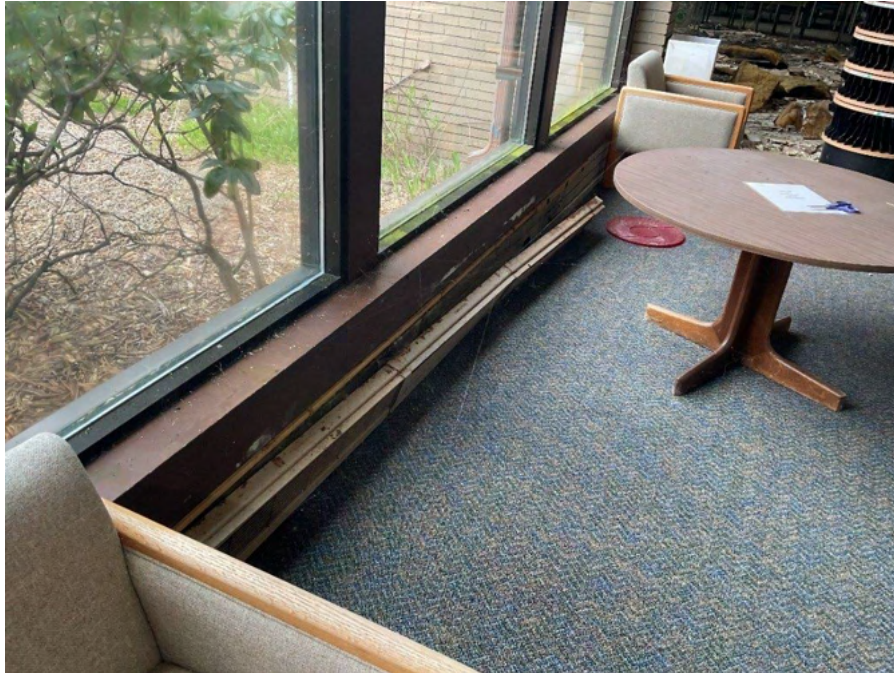
Main Floor – Heating panel damage (Photo No. 4876)
