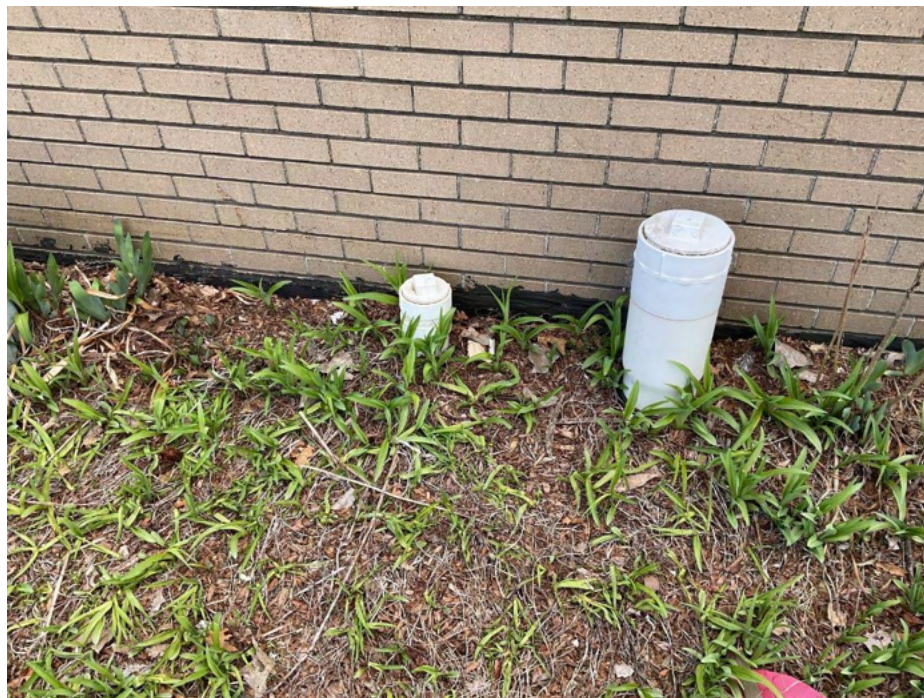
Exterior Area – Depression area, lack of positive drain (Photo No. 5049)
