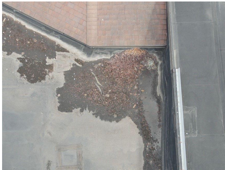
Flat Roof – Water ponding/ Lack of positive drain (Parking Lot Side Photo No. 56)
