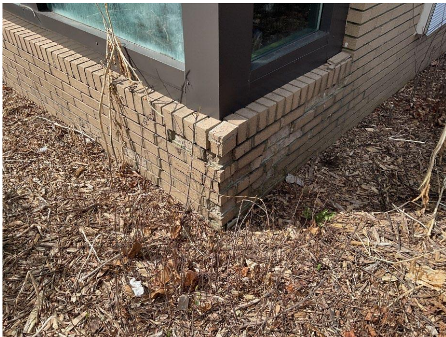
External Area – Brick damage (Photo No. 5031)
