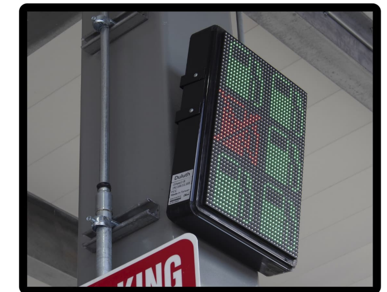
FUEL INDICATOR LIGHT SYSTEM
