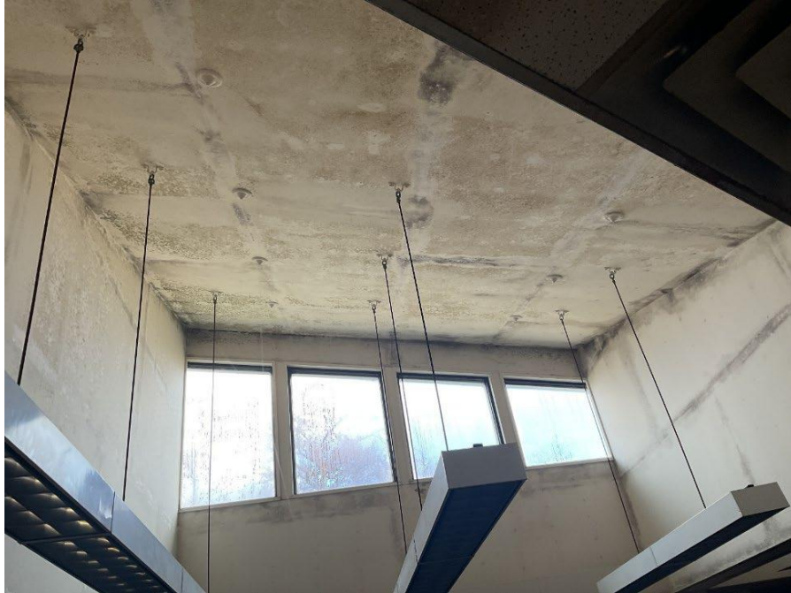
Main Floor – Ceiling mold (Photo No. 4911))
