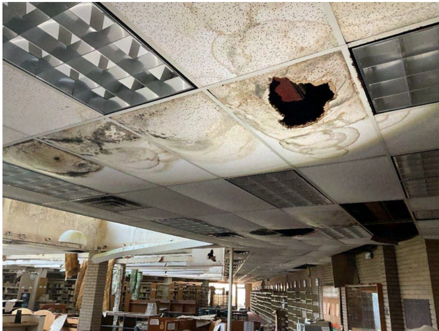
Main Floor Ceiling – Typical water damage (Photo No. 4838)
