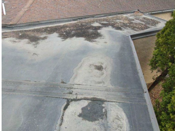
Flat Roof – Damage at the curb connecting to shingle roof, lack of positive drain (Parking Lot Side Photo No. 23)
