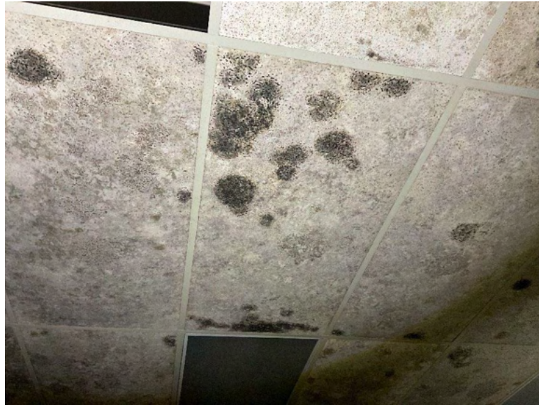
Basement Ceiling – Mold (Photo No. 4682)
