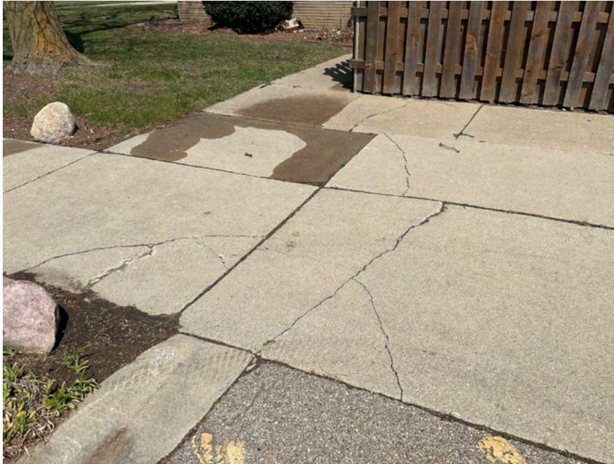
Exterior area: walkway concrete damage (Photo No. 5055)
