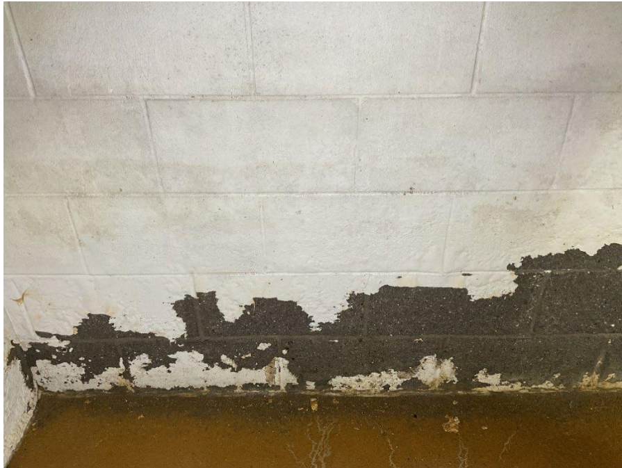
Basement Wall - Paint damage and mold (Photo No. 4718)
