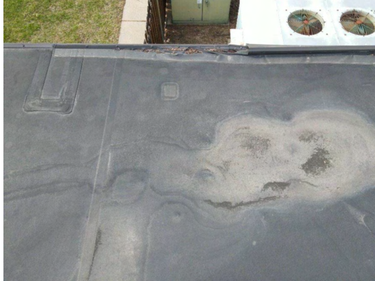
Flat Roof- Damage at edge (Parking Lot Side Photo No. 51)
