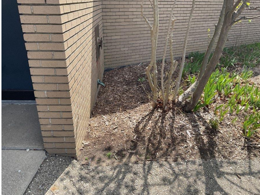
External Area – Depression area, lack of positive drainage (Photo No. 5048)
