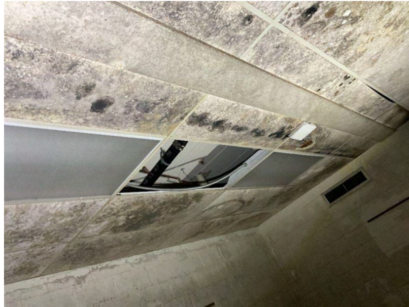
Basement – Ceiling panel missing (Photo No. 4684)
