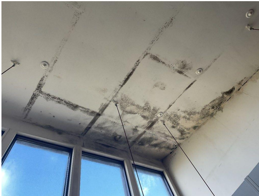
Main Floor Ceiling - Mold (Photo No. 4852)
