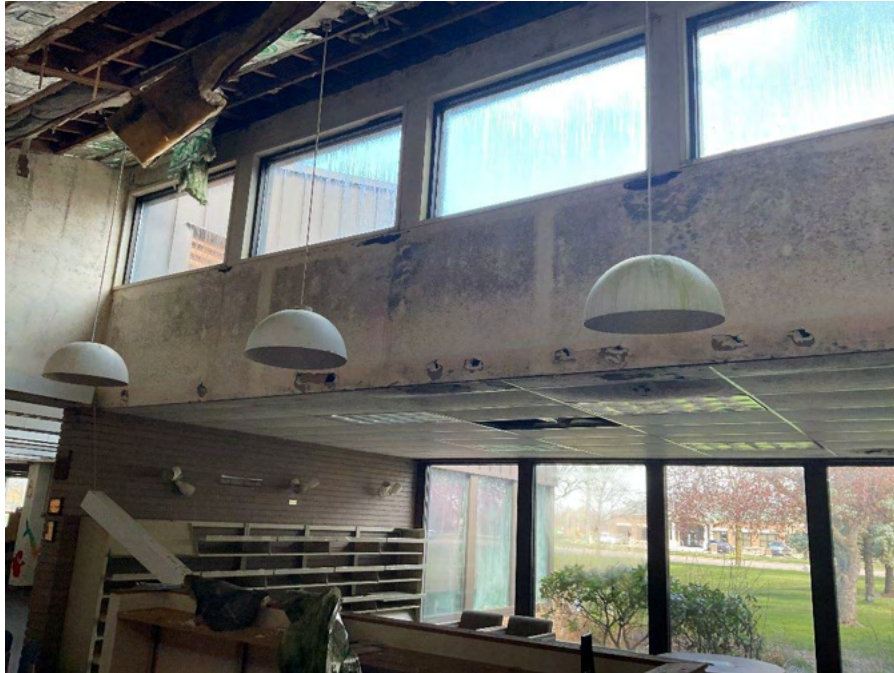
Main Floor – Moisture in windows (Photo No. 4981)
