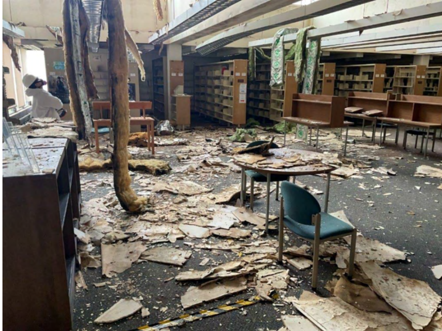
Main Floor – Floor Conditions (Photo No. 4885)
