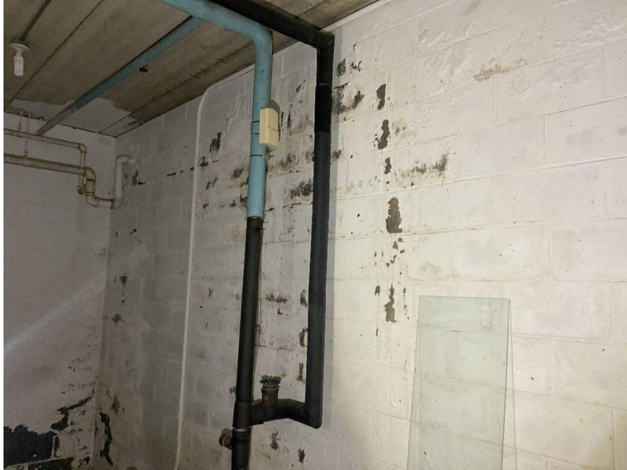
Basement Wall Mechanical Room – Water infiltration through wall (Photo No. 4716)
