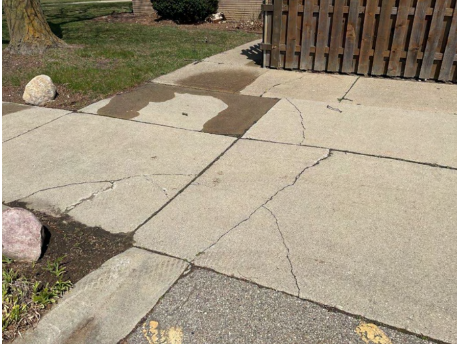
Exterior area: walkway concrete damage (Photo No. 5055)
