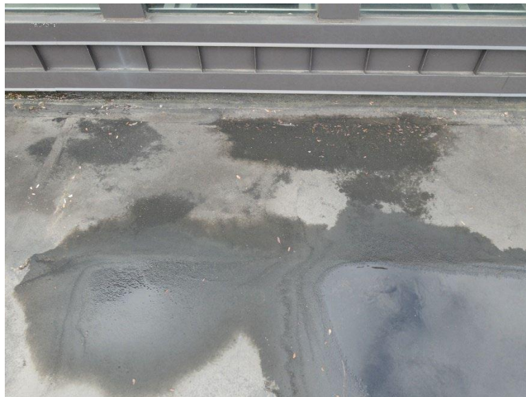
Flat Roof -Water ponding (Plymouth Rd Photo No. 71)
