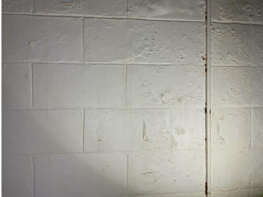
Basement wall – Moisture Infiltration (Photo No. 4688)
