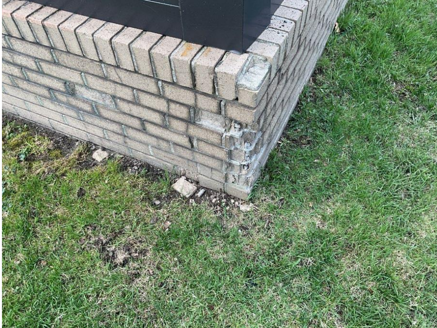
External Area – Brick damage (Photo No. 5030)
