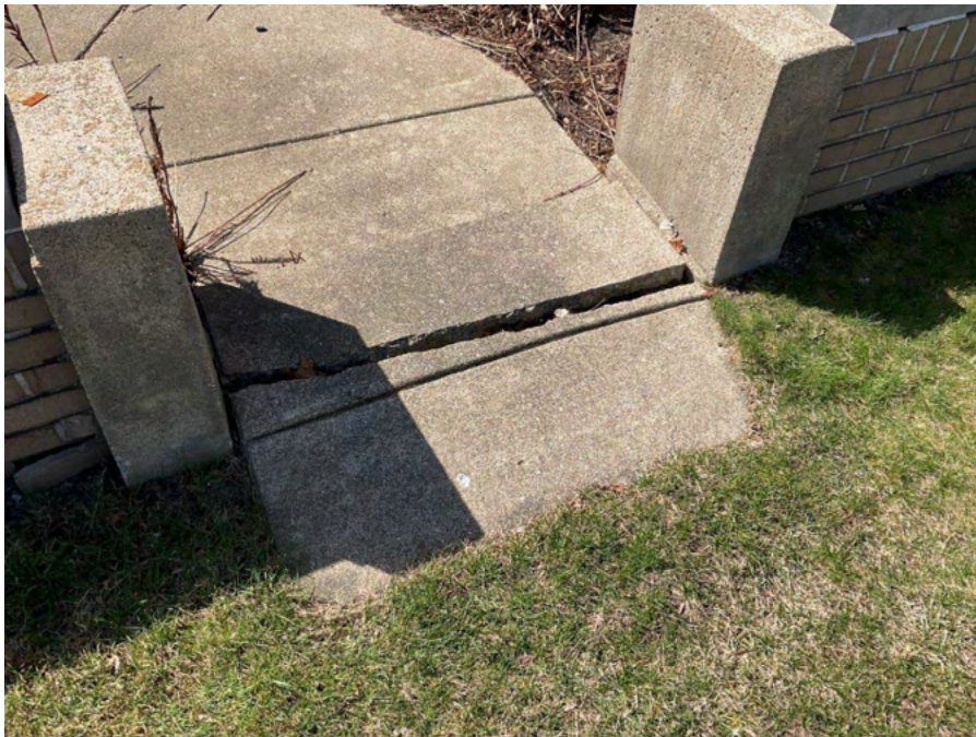
External Area – Concrete damage (Photo No. 5038)
