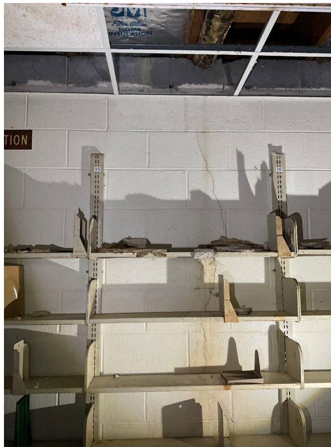
Main Floor Adult Reading Room – Wall crack (Photo No. 4921)
