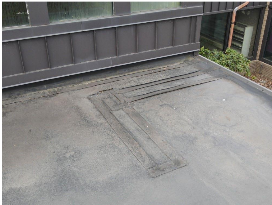
Flat Roof – Damage of patching repair (Plymouth Rd Photo No. 29)
