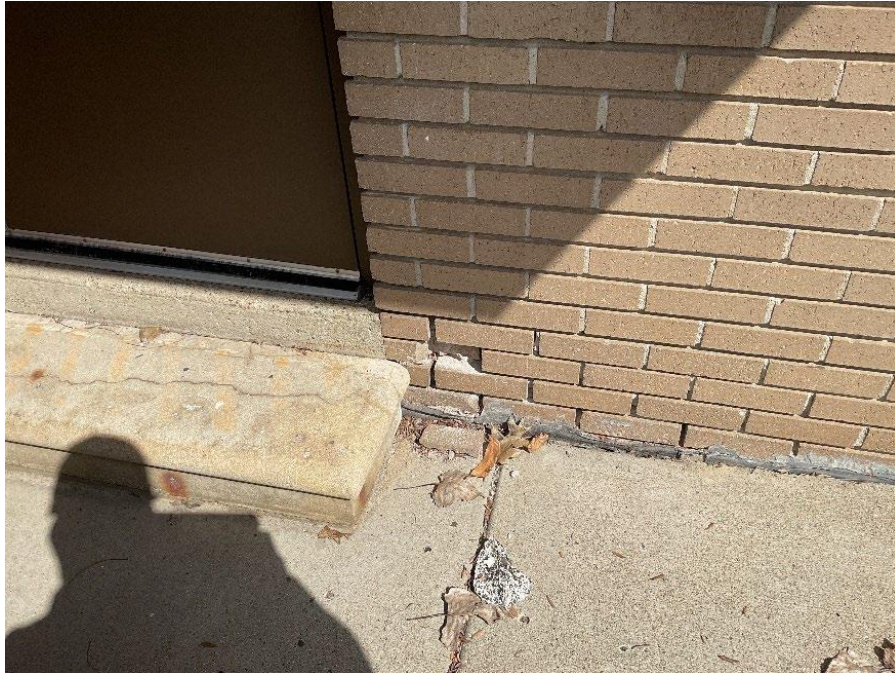
Exterior Wall - Brick damage (Photo No. 5005)
