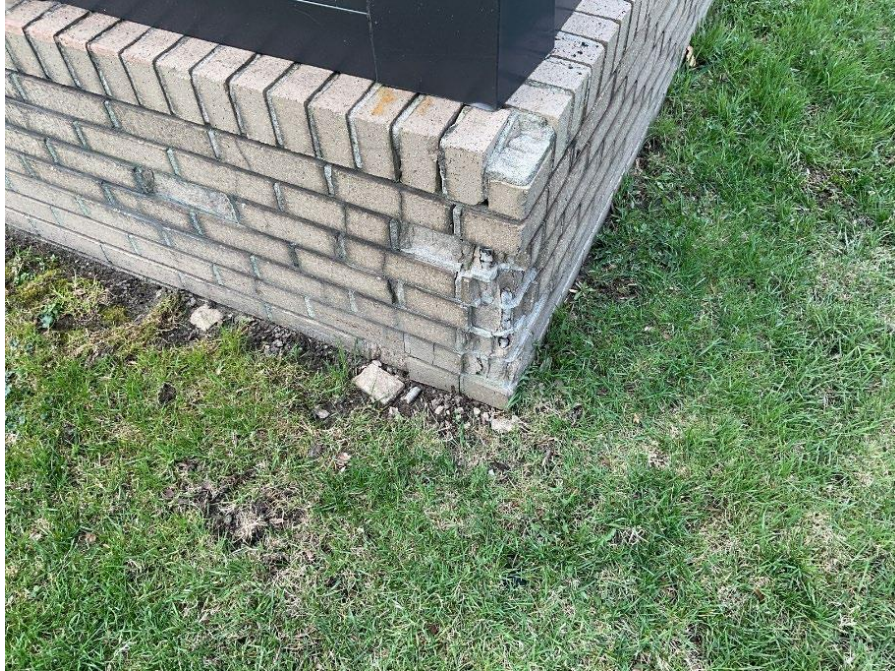
External Area – Brick damage (Photo No. 5030)
