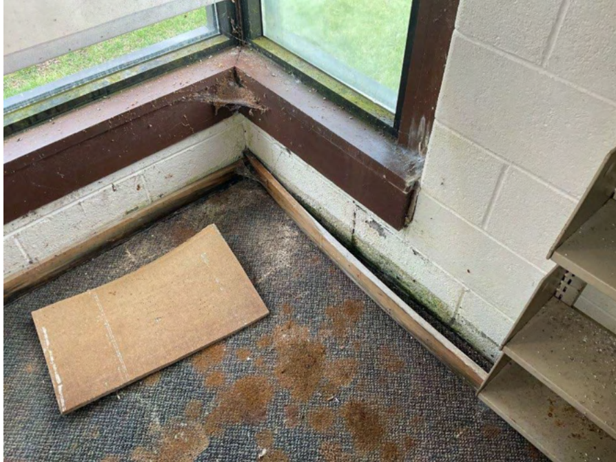
Main Floor – Kicker plate damage (Photo No. 4897)
