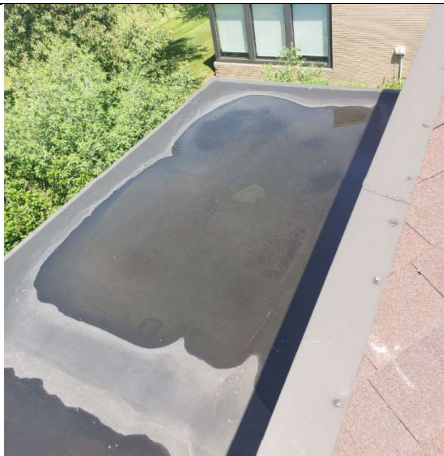
Roof ponding, little/no positive slope to scuppers
