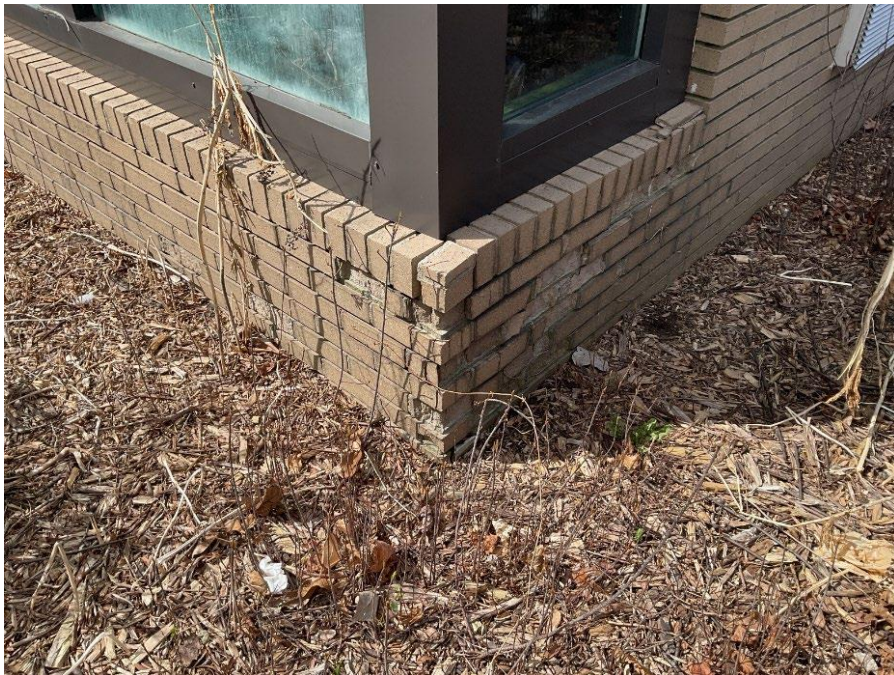
External Area – Brick damage (Photo No. 5031)
