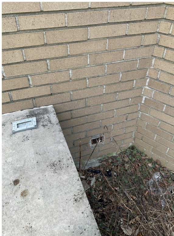
Electrical Outlet – Loose cover (Photo No. 5020)
