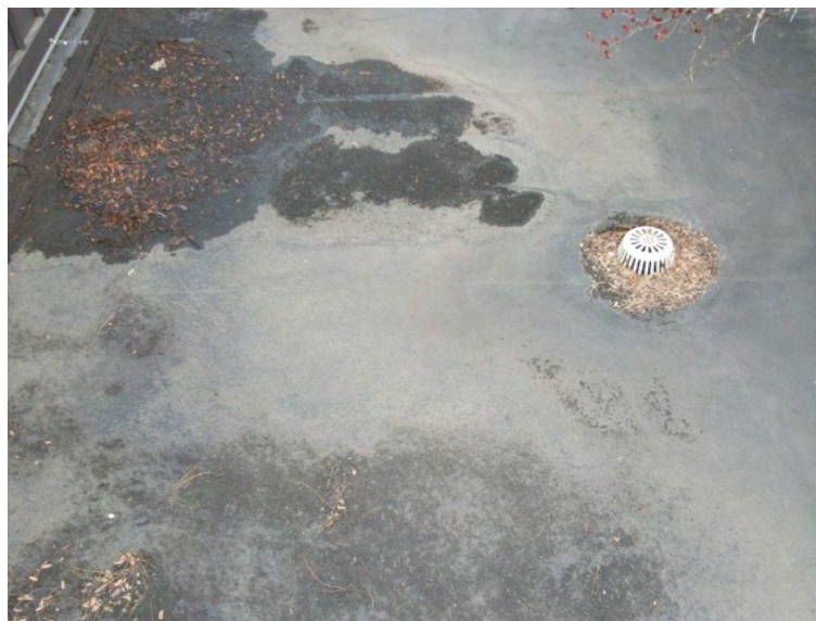
Flat Roof – Lack of positive drain (Parking Lot Side Photo No. 20)
