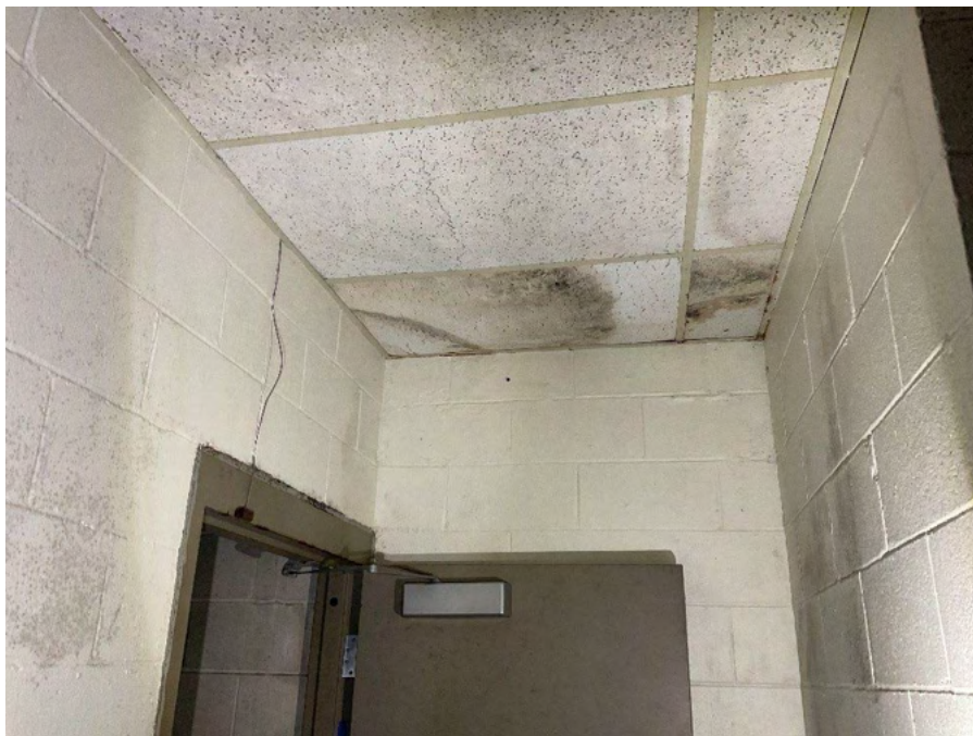
Basement Ceiling – Water infiltration from first floor (Photo No. 4696)
