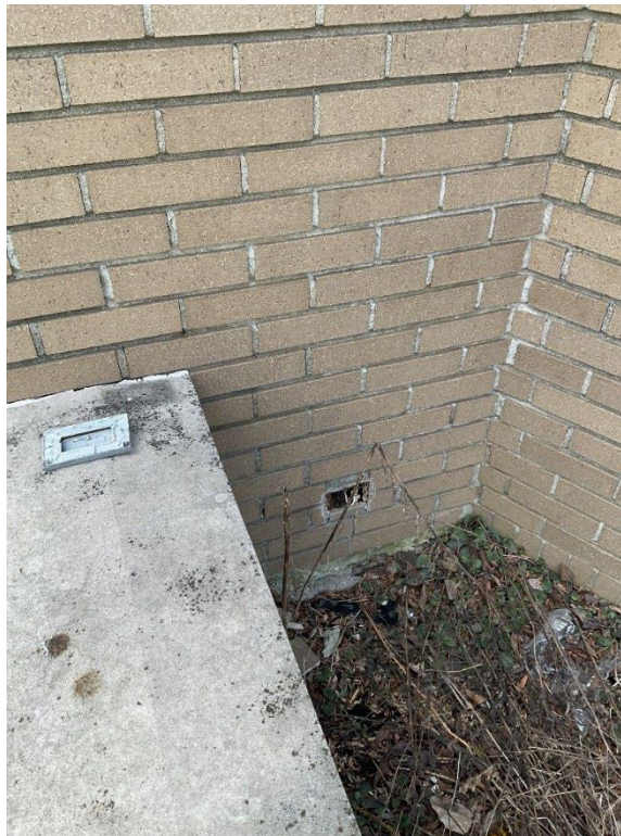
Electrical Outlet – Loose cover (Photo No. 5020)
