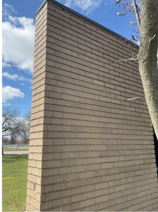
Exterior Wall – Brick damage (Photo No. 5018)
