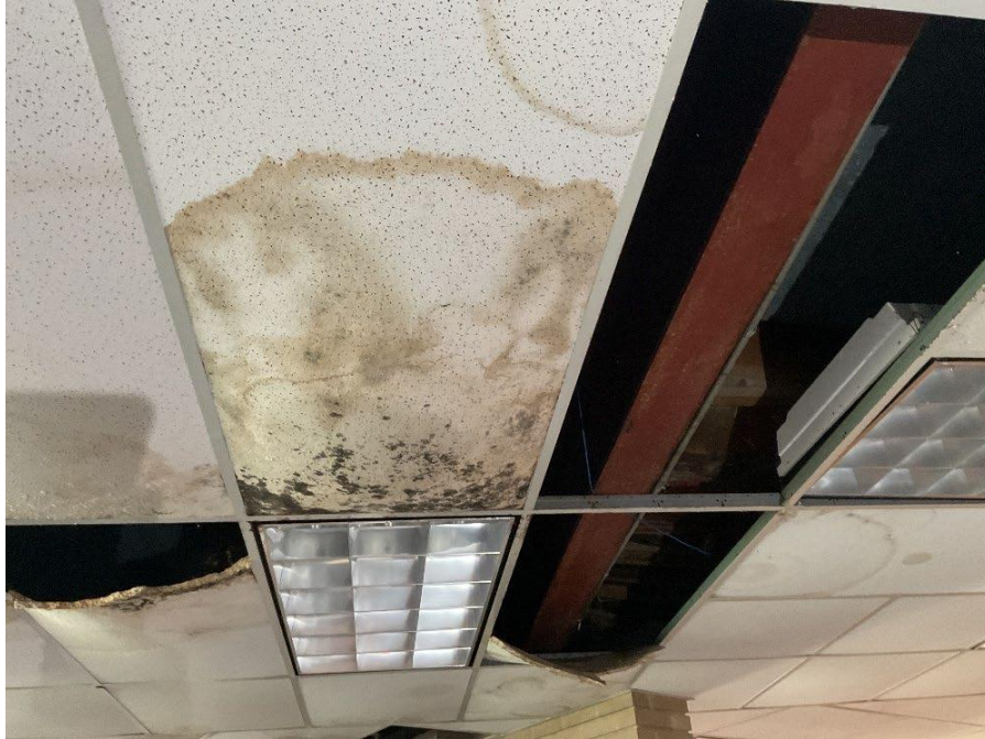
Main Floor – steel beam corrosion (Photo No. 4840)
