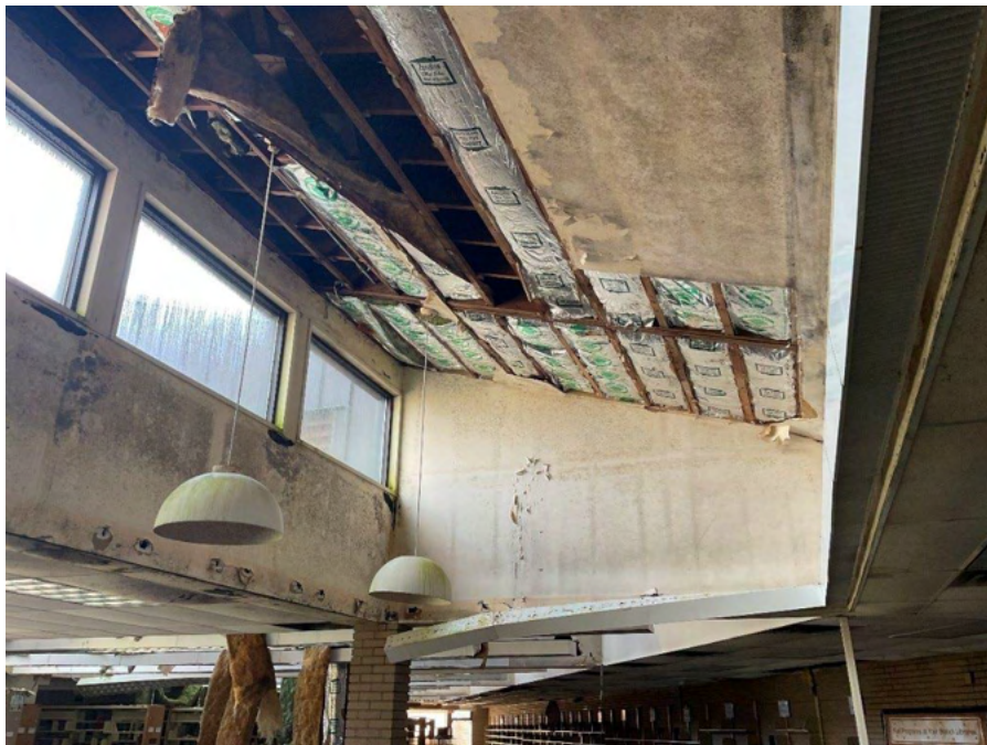
Main Floor Lounge – Ceiling damage/Insulation damage/ mold on wall (Photo No. 4863)
