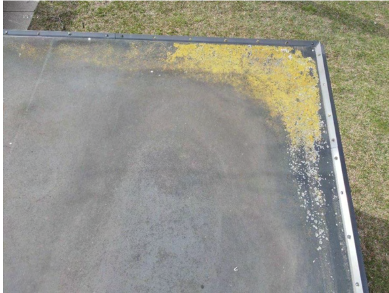
Flat Roof – Lack of positive drain (Woodring Ave Photo No. 2)
