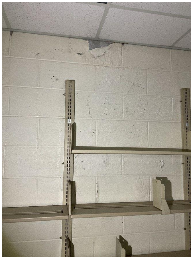
Main Floor Wall – Water damage (Photo No. 4848)
