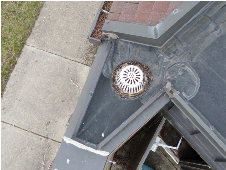
Flat Roof – Potential drain inlet clog (Plymouth Rd Photo No. 23)
