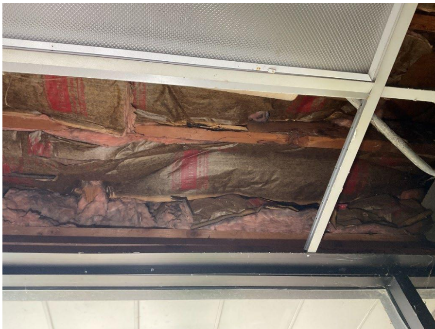
Basement Ceiling – Damage insulation with mold (Photo No. 4754)
