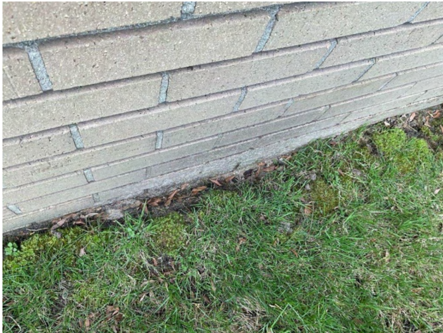
External Area – Local depression area due to drainage (Photo No. 5029)
