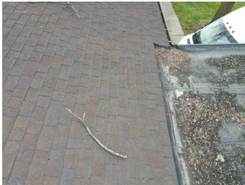
Shingle Roof – Damaged shingle piece (Loveland St and Parking Lot Photo No. 47)
