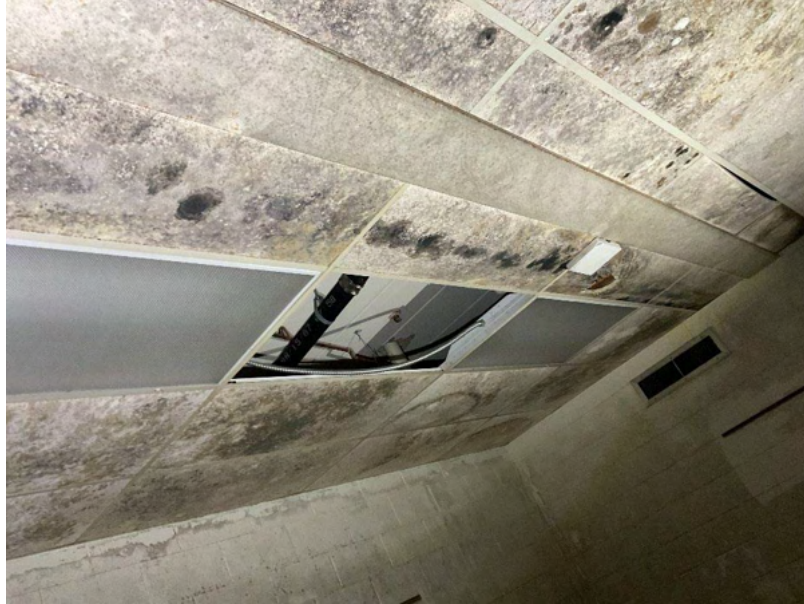
Basement – Ceiling panel missing (Photo No. 4684)
