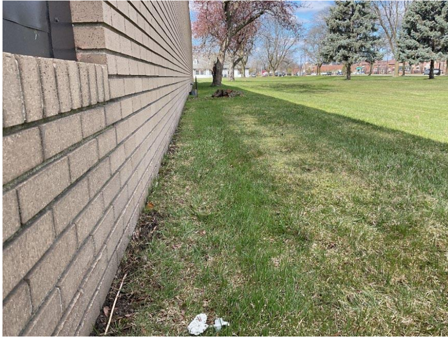
External Area - Evidence of water seepage at toe of wall (Photo No. 5025)
