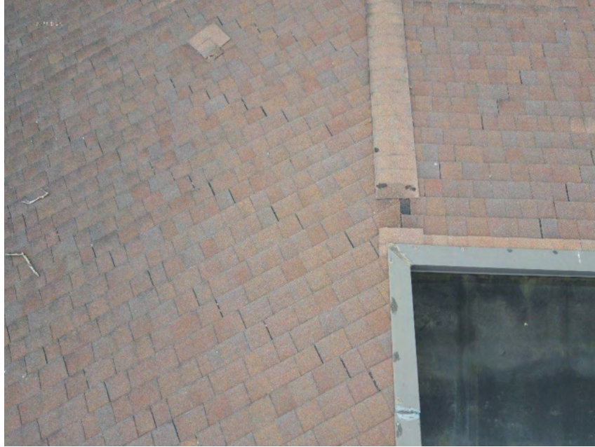
Shingle Roof – Loose shingle piece (Loveland St and Parking Lot Photo No. 39)
