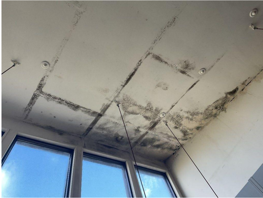
Main Floor Ceiling - Mold (Photo No. 4852)
