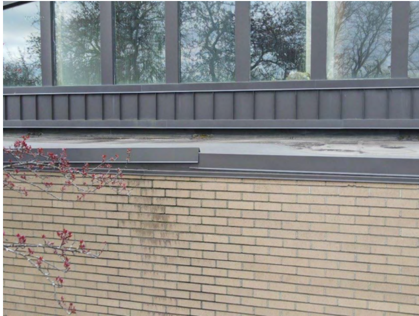
Roof – Loose flash panel (Plymouth Rd Photo No. 24)
