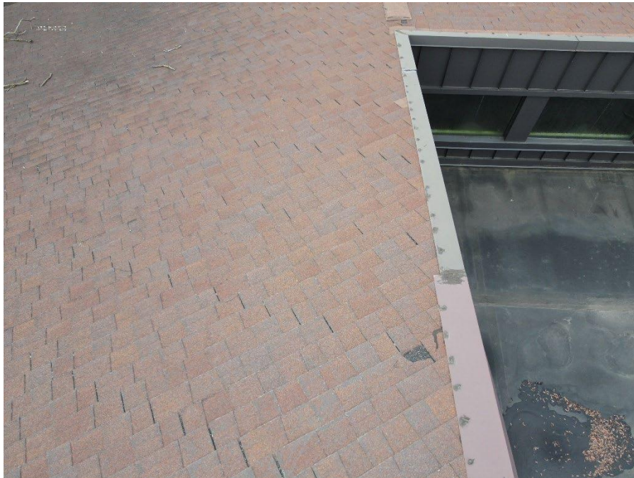
Shingle Roof – Damaged shingle (Loveland St and Parking Lot Photo No. 37)
