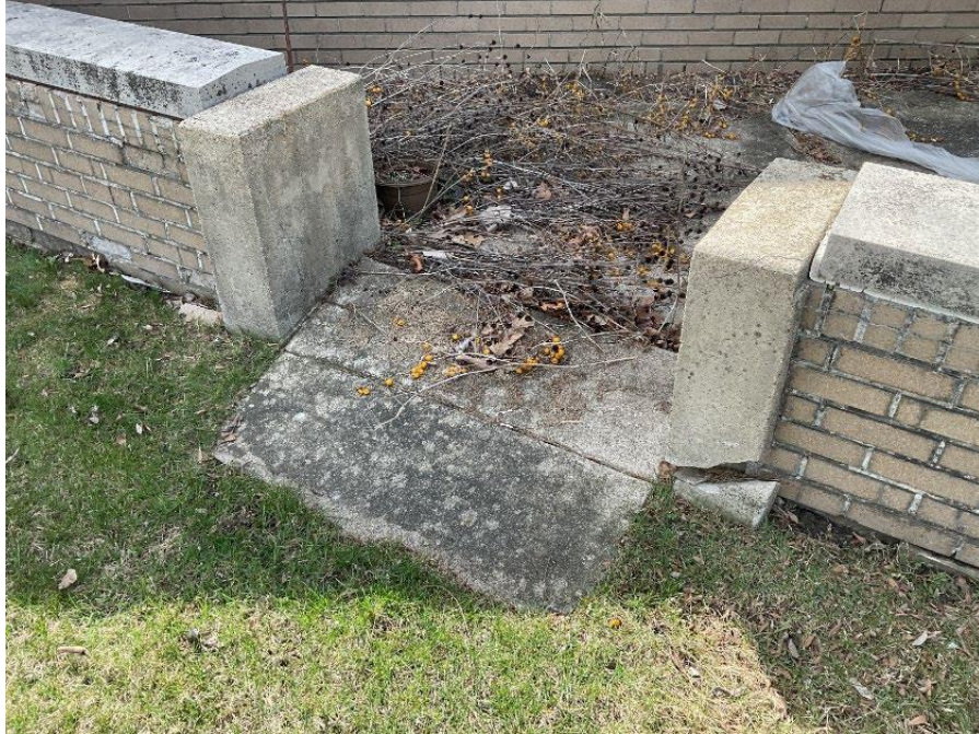
External Area – Concrete damage (Photo No. 5021)
