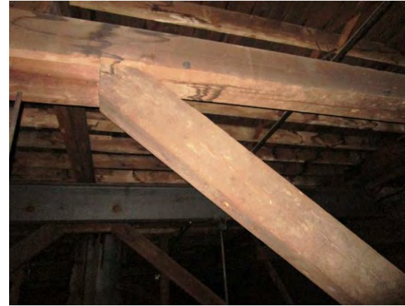
Figure 39 - View of the longitudinal cracking and splitting of the top chord and members below the cupola.
